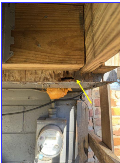
Damaged under deck
