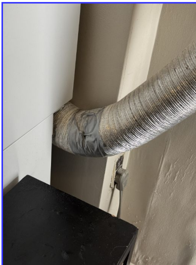
Incorrect repair at laundry
