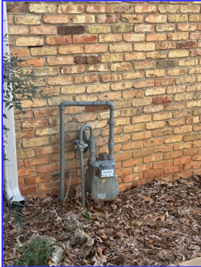
Gas meter at the right side
