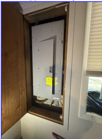
Main panel box located in the Basement
