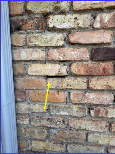
Damaged brick and mortar at home
