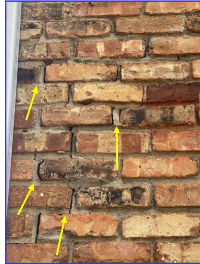
Cracked brick siding at rear
