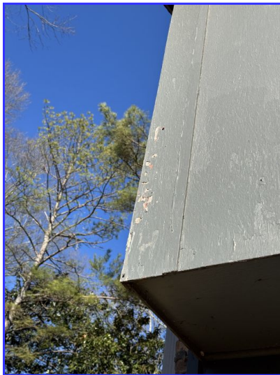
Common cracks/chips noted at the corners of the siding.
