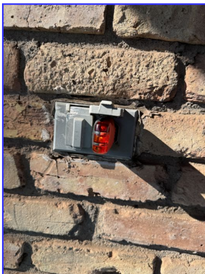
no gfci at exteriors
