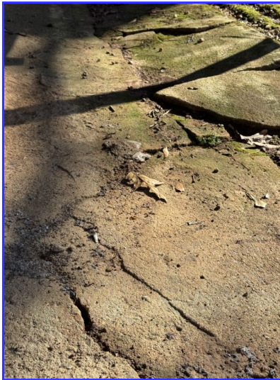
Erosion under deck
