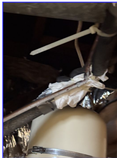
Incorrect repair a lines
