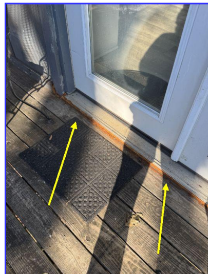
Incorrect repair at deck
