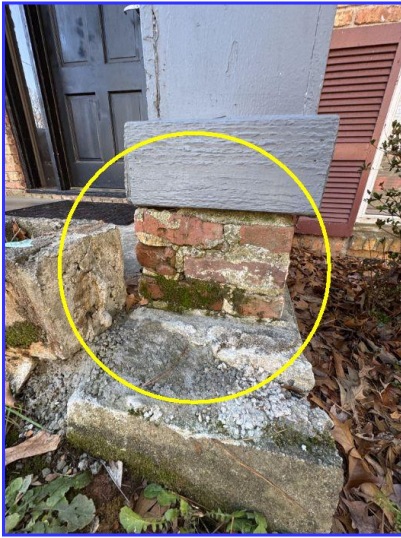
Damaged pillars at porch
