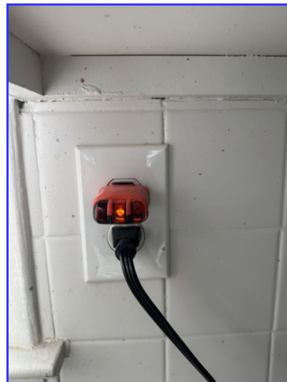
no grounding or gfci at kitchen
