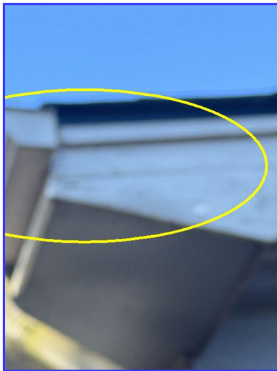
Damaged trim at rear
