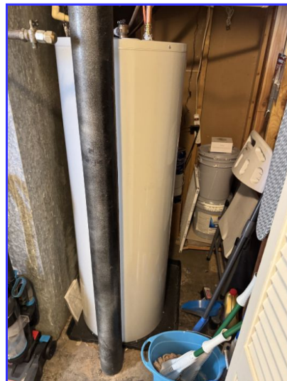
Water heater located in the basement
