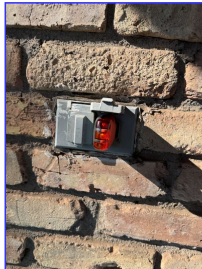
No gfci at exterior outlets
