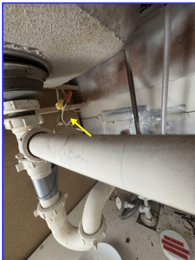
Open wires under kitchen sink
