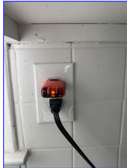
no grounding or gfci at kitchen
