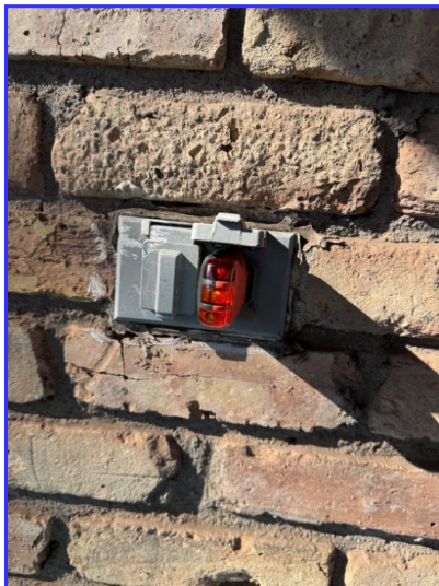
no gfci at exteriors
