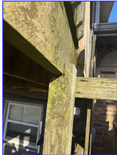
Missing straps and bolts
