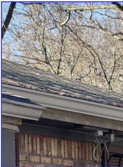
Gutters are clogged around the home
