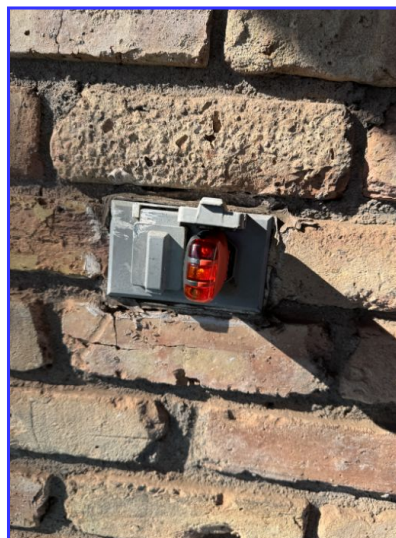
No gfci at exterior outlets
