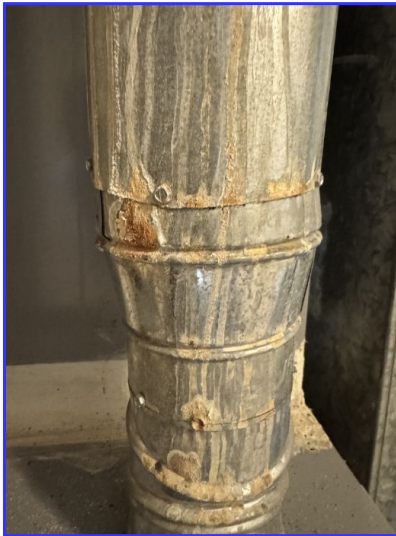
Rust noted on metal vent pipe
