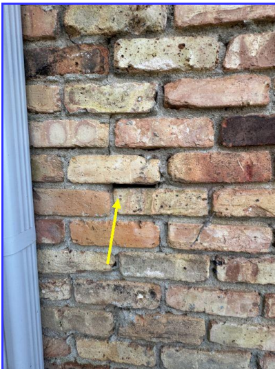
Damaged brick and mortar at home
