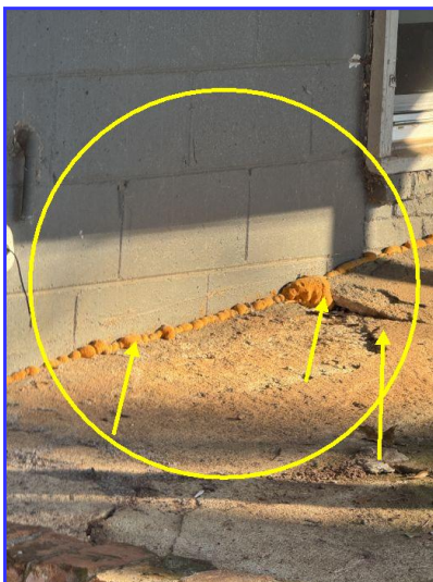
Incorrect repair at rear foundation
