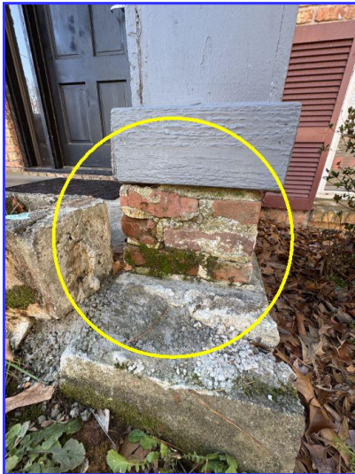
Damaged pillars at porch
