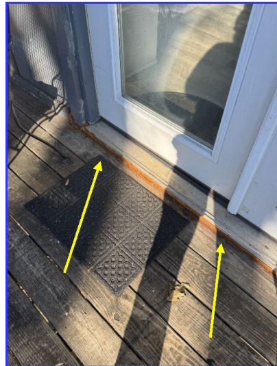
Incorrect repair at deck
