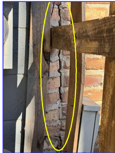
Damaged brick and mortar at rear
