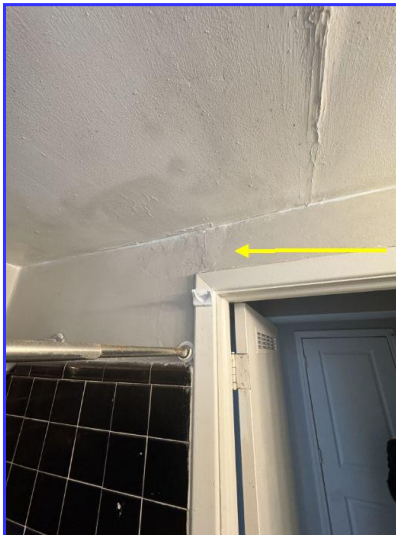
Damaged wall at bathroom
