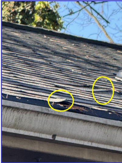
Curling noted on shingles on roof
