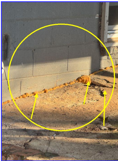
Incorrect repair at rear foundation
