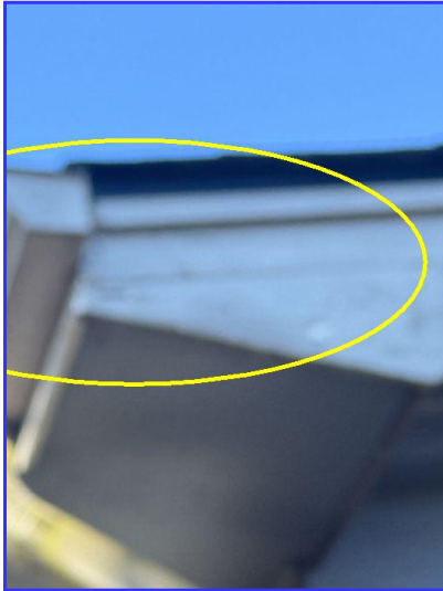
Damaged trim at rear
