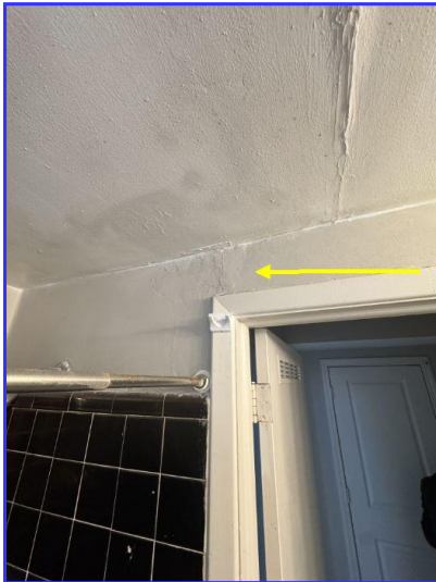
Damaged wall at bathroom
