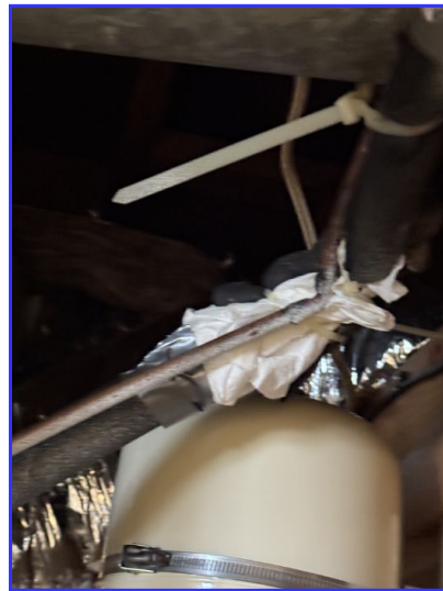
Incorrect repair a lines
