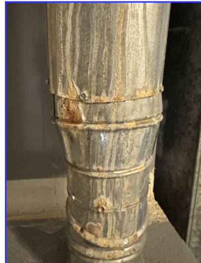
Rust noted on metal vent pipe
