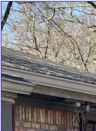
Gutters are clogged around the home
