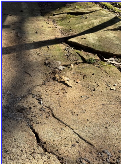
Erosion under deck
