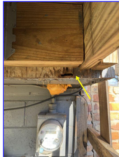
Damaged under deck
