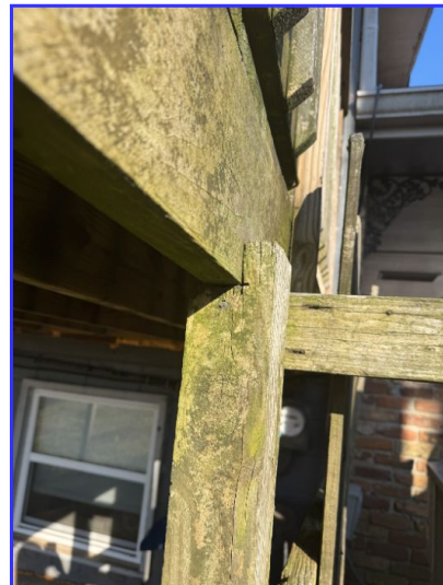
Missing straps and bolts
