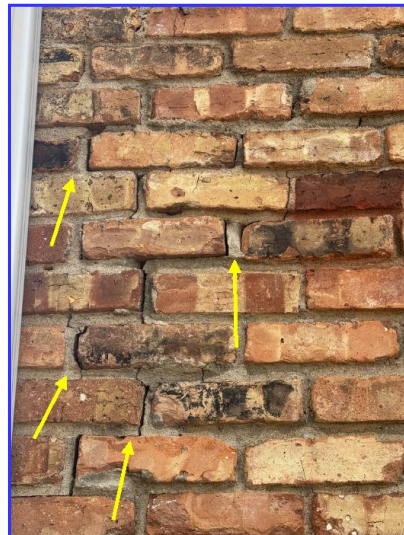
Cracked brick siding at rear
