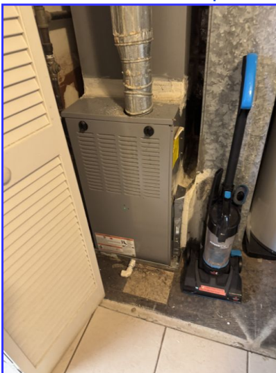
Furnace located in basement
