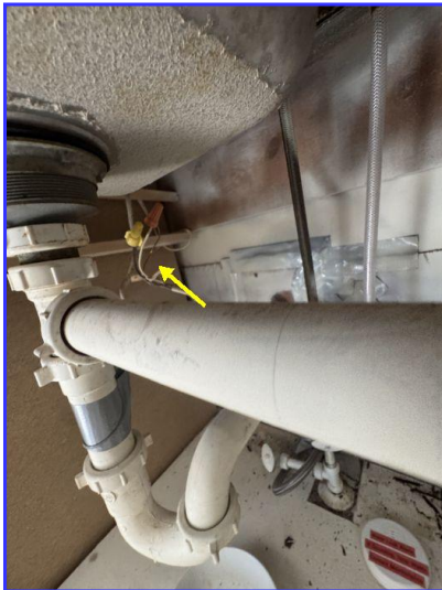
Open wires under kitchen sink
