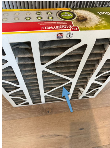
Air filter at air handler needs to be replaced
