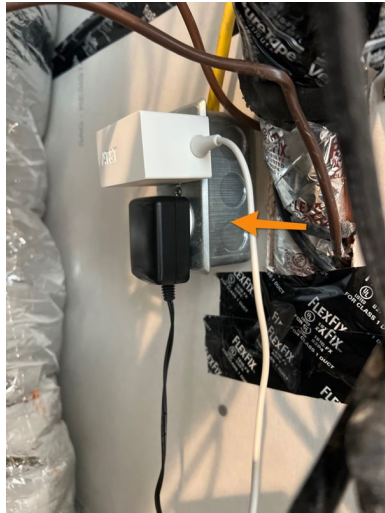
Air handler closet
