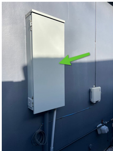
Main electrical service panel
