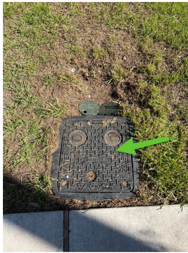
Water meter box
