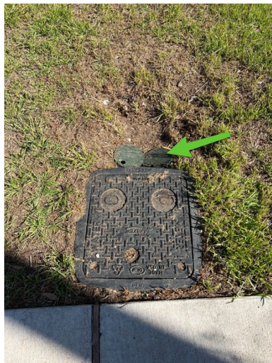
Main water shut off box
