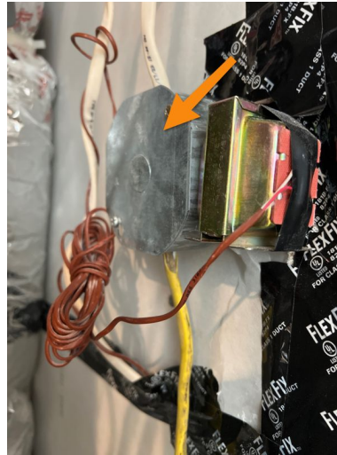
Air handler closet
