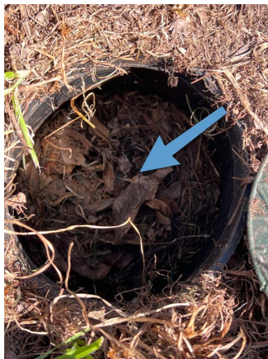
Pressure reducing valve is buried
