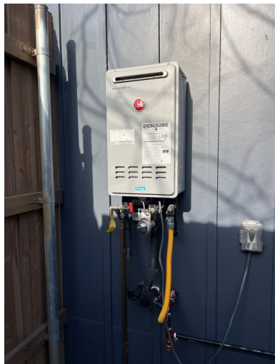
Tankless water heater located right side of home
