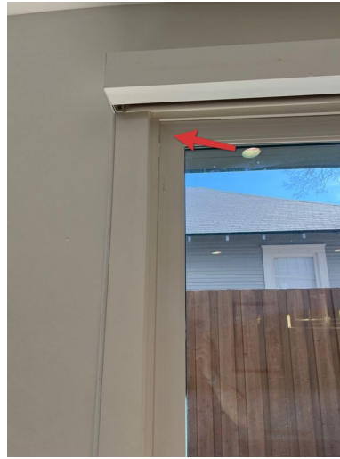
Missing door alarm
