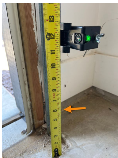
Garage opener safety sensors are too high
