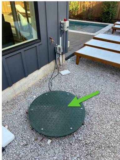
Sewage grinder pump, not part of inspection
