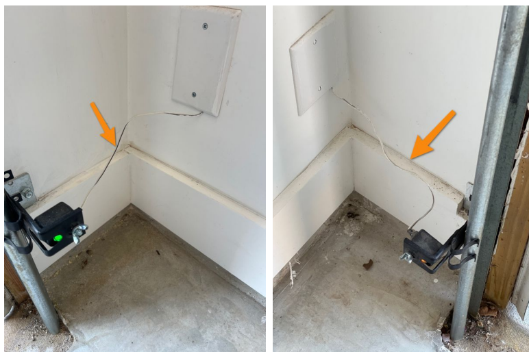
Sensor wires should be secured to wall
