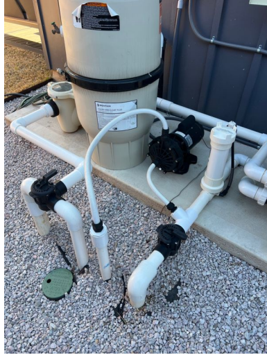
Missing paint on PVC pipes
