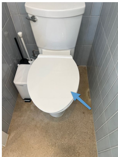
Loose toilet at downstairs half bathroom
