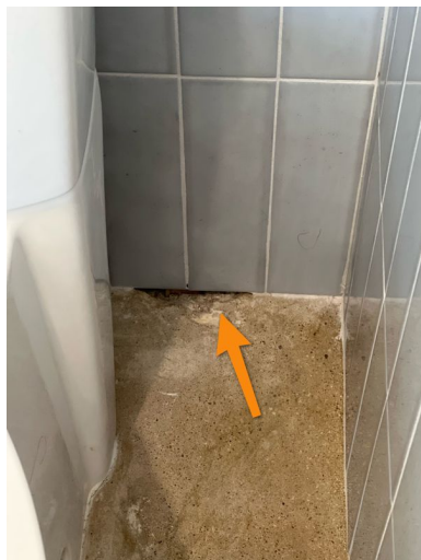
Behind toilet at downstairs half bath
