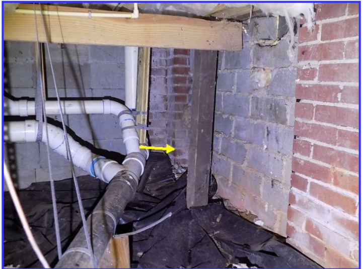
Leaning support at right wall
