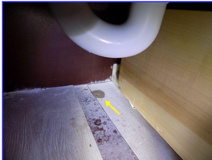
Leak at drain under sink in the main level guest bath
