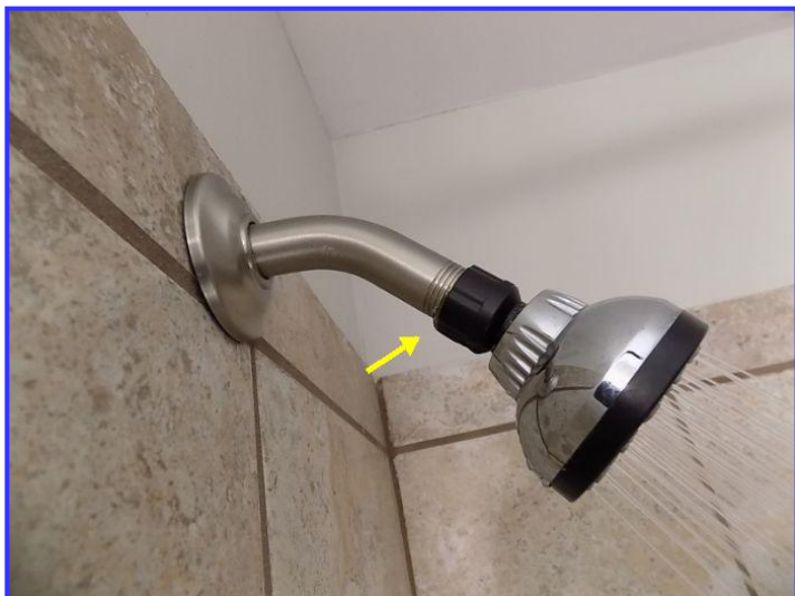
Leak at shower faucet at upstairs hall bath
