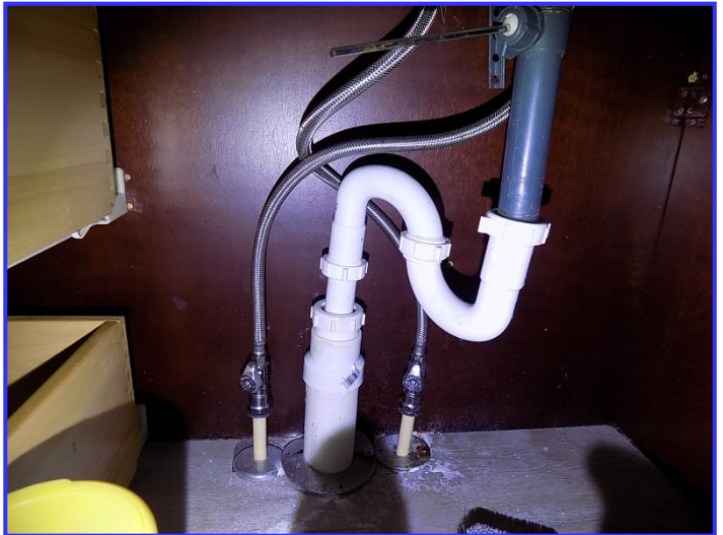
S Trap at upstairs hall bath
