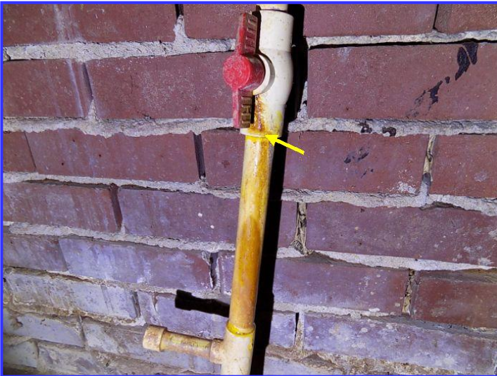
Leak noted at main water shutoff
