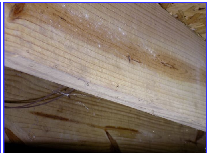
Organic growth on framing
