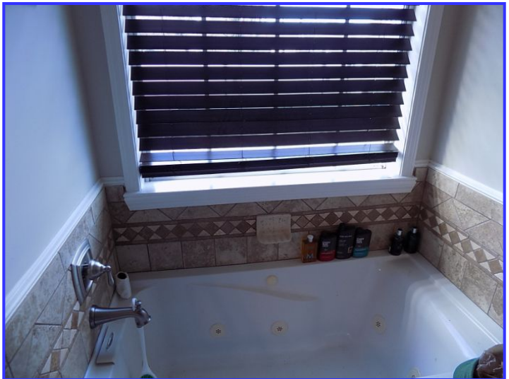
No safety glass over master bath tub
