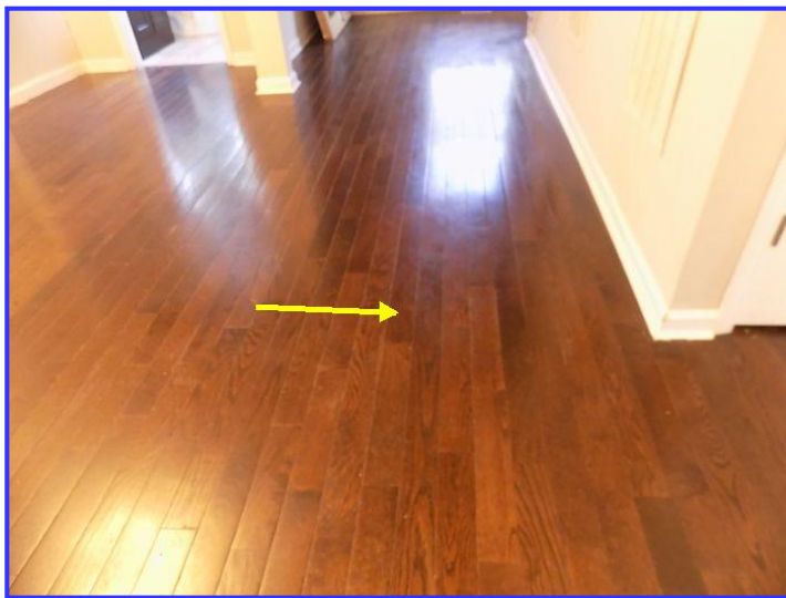
Low spot in floor at main foyer
