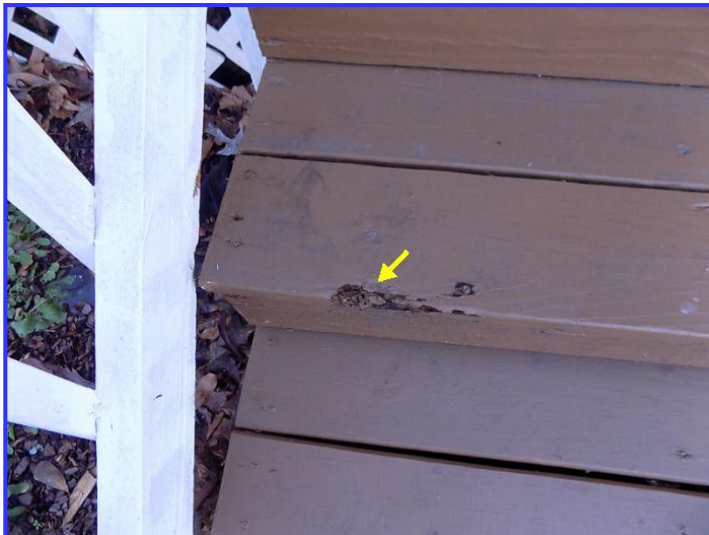
Damaged tread at front porch stairs
