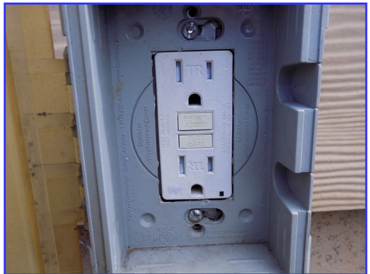
GFCI will not trip when re set at right
