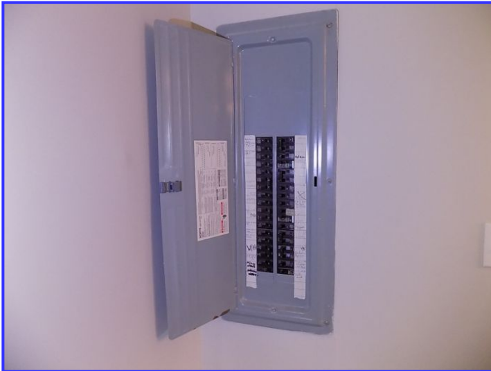
Main panel located in hallway
