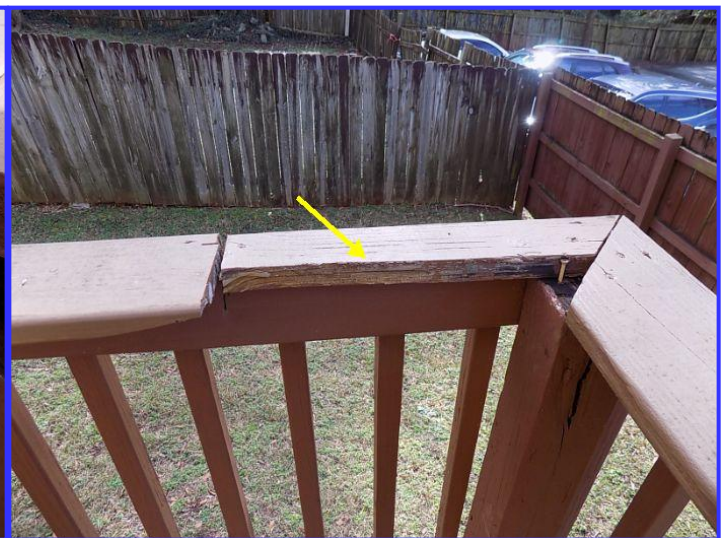
Damaged handrail at rear deck
