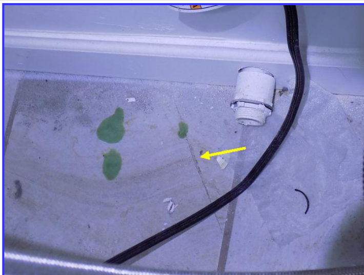
Cracked tiles at laundry room
