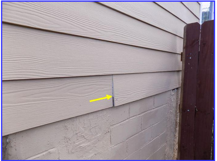
Loose siding at right
