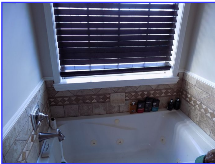
No safety glass over master bath tub
