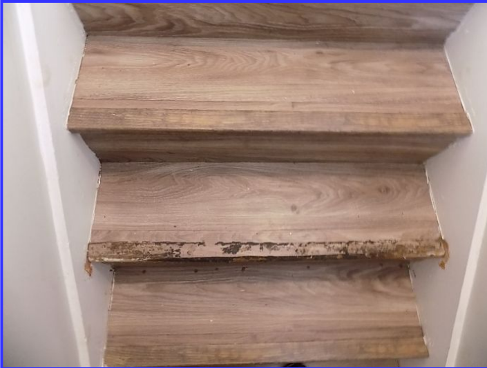
Damage at stars
