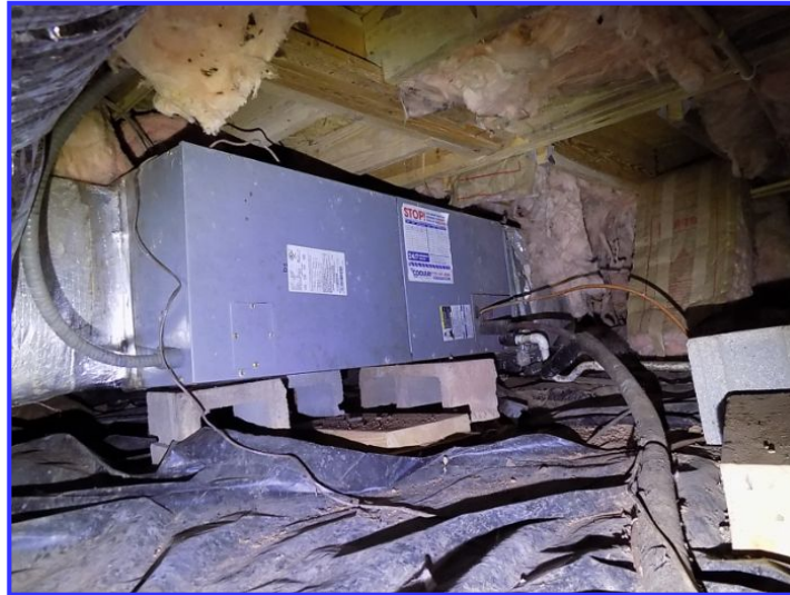
Furnace in crawlspace
