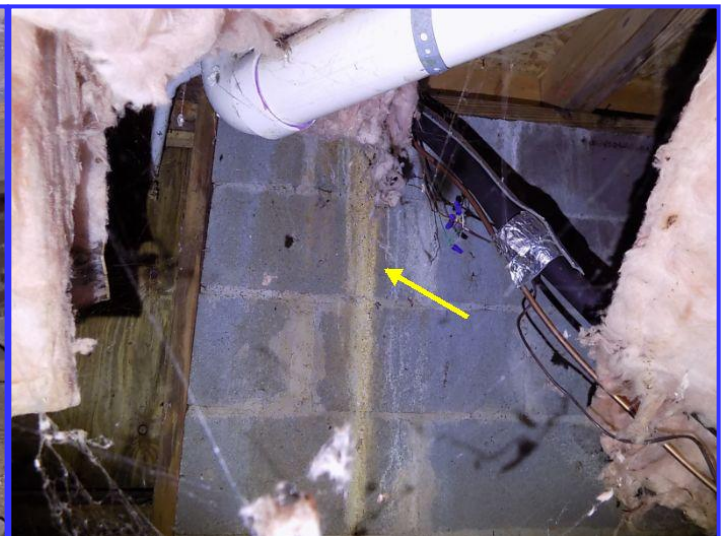
Efflorescence noted at rear wall
