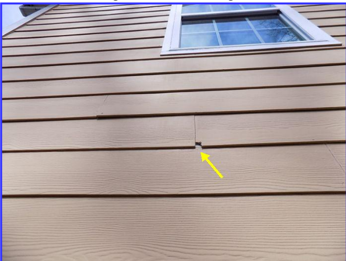
Damaged area of siding at rear
