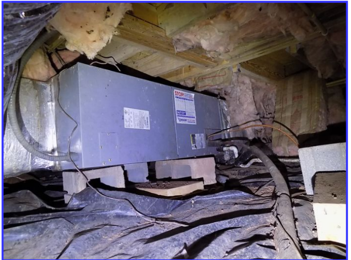
Furnace in crawlspace
