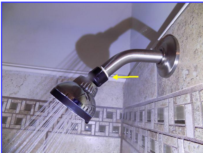
Leak at main level guest bath shower
