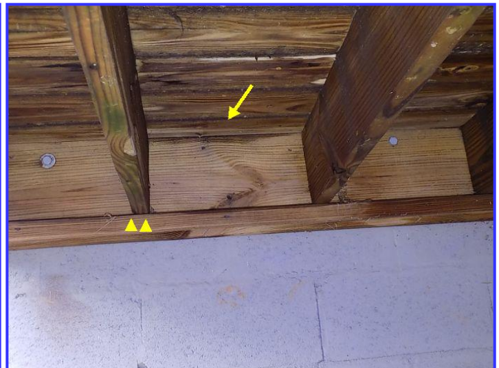
No flashing between deck and home, 3 nails needed
