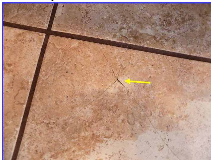
Cracked tiles at kitchen
