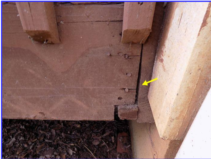
Separation at band at rear deck
