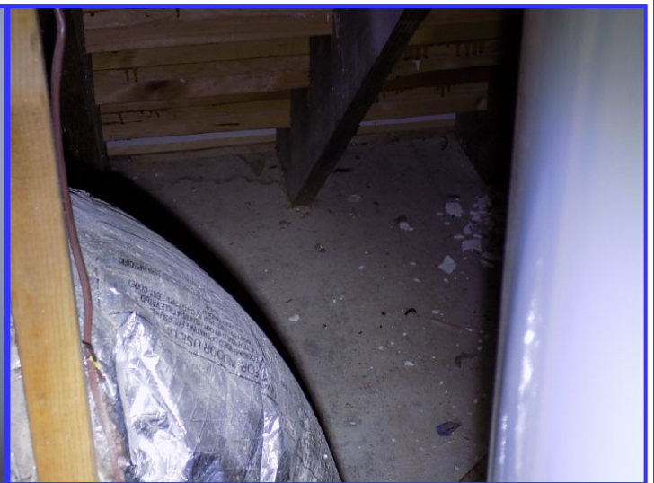
Rodent droppings under stairs at main level
