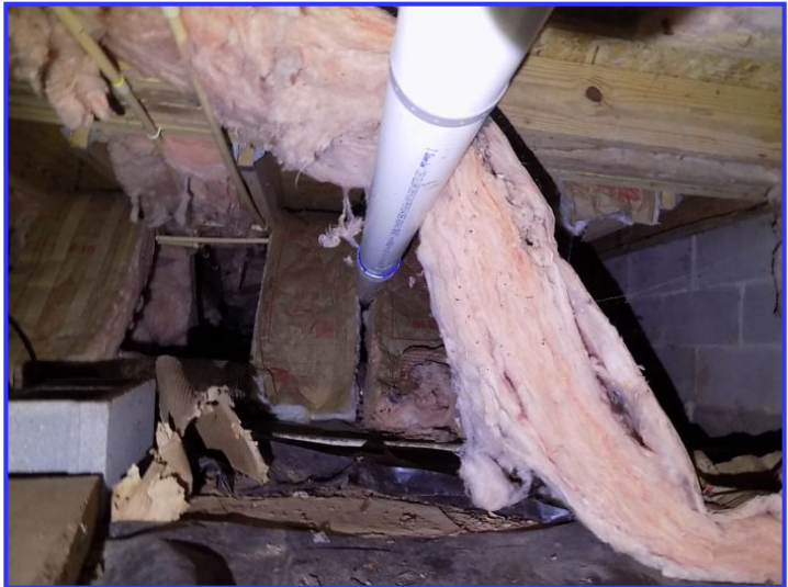
Limited view at rear wall due to fallen insulation
