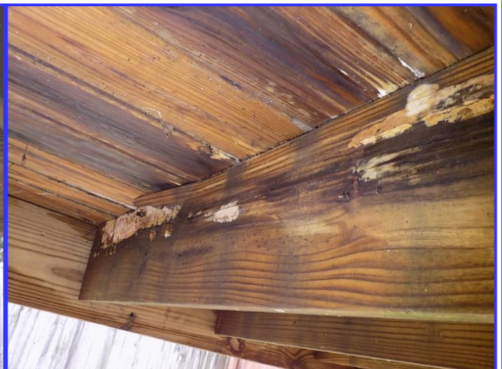
Wood rot at multiple deck joists
