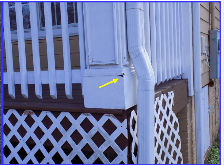
Damaged support post at front porch
