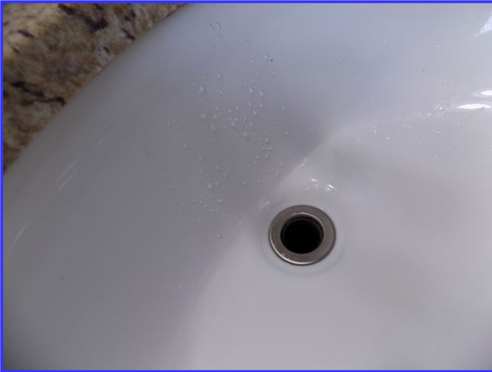
Non functioning drain stopper noted at the upstairs hall bath
