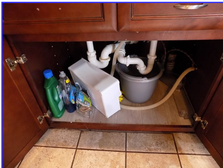
Limited view beneath sink due to storage
