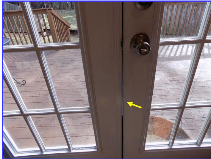
Gap at weatherstripping at rear door
