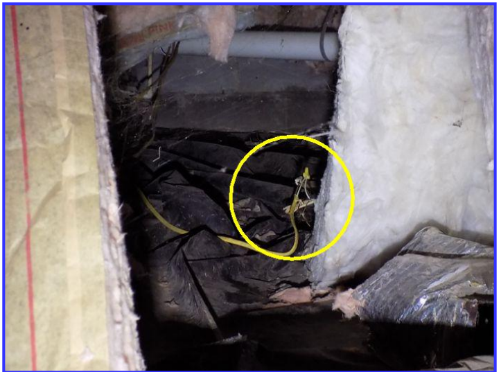
Open splices at rear crawlspace wall
