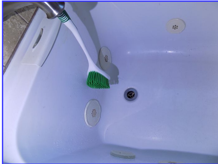
Missing plug at master bath, unable to test jets
