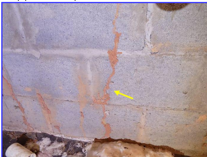
Possible termite activity at right wall
