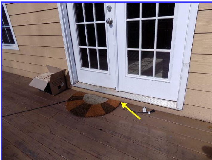
Suggested to install blocking under the threshold at exterior doors.
