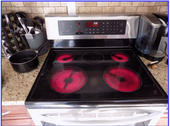
No anti tip bracket installed at stove
