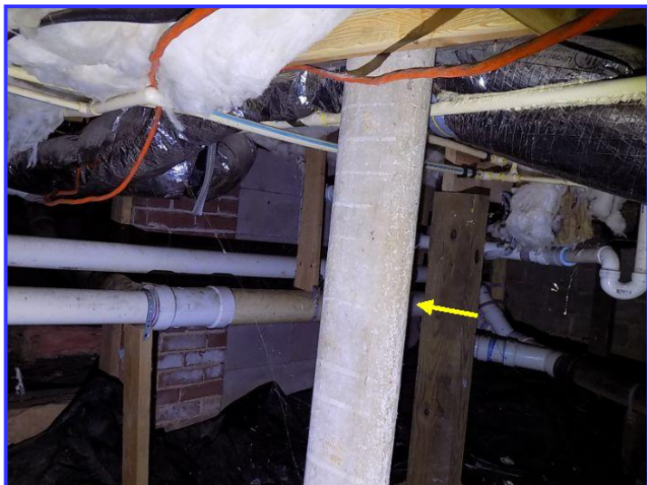
Possible asbestos transite pipe in crawlspace
