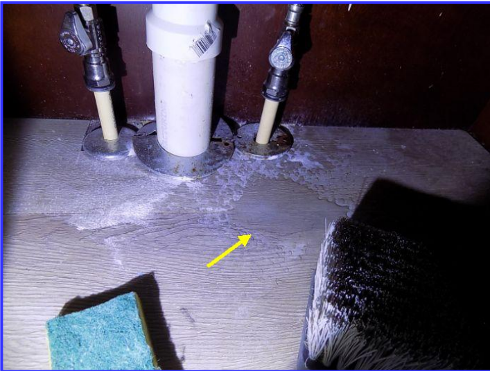
Leak at drain under sink in the upstairs hall bath
