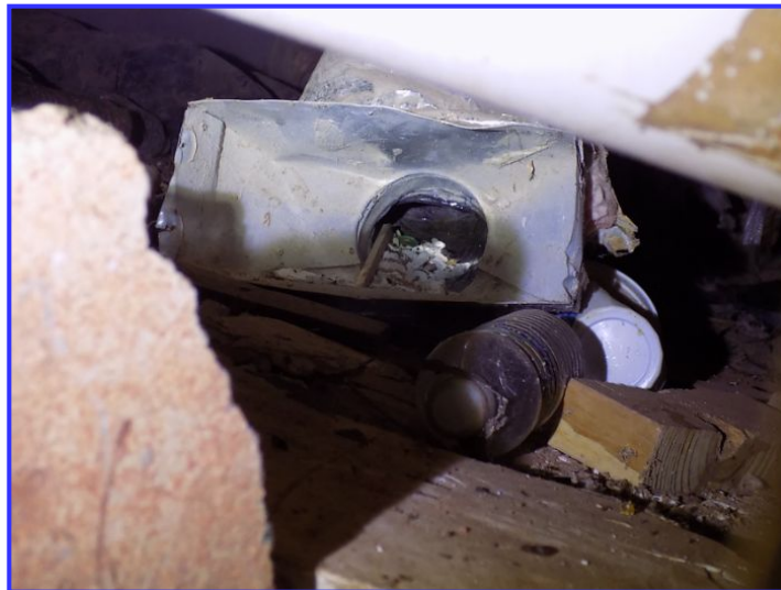
Disconnected duct at left wall
