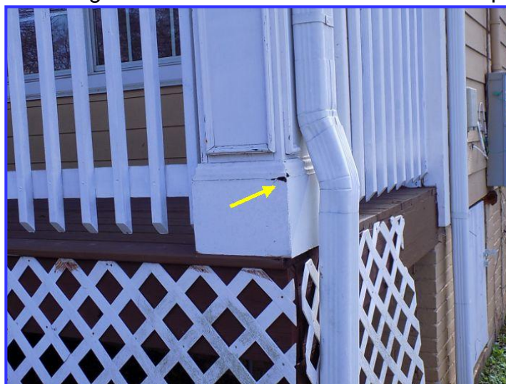
Damaged support post at front porch
