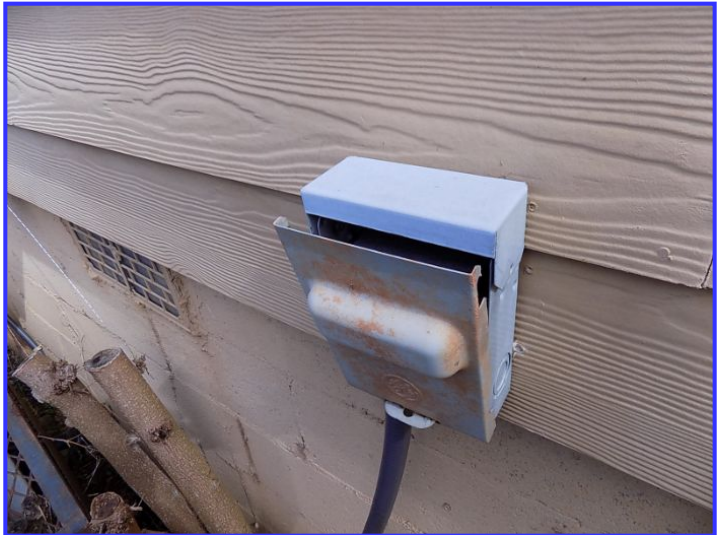
Loose cover at AC disconnect
