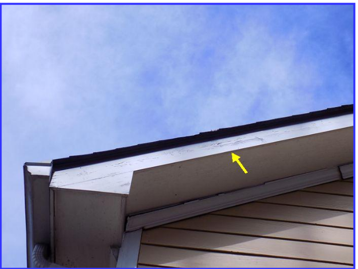
Weathered fascia at rear
