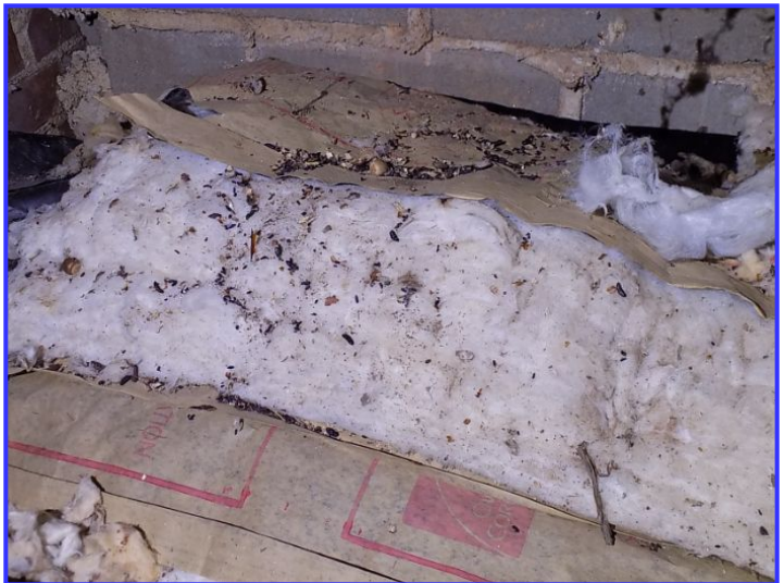
Rodent contaminated insulation in crawlspace
