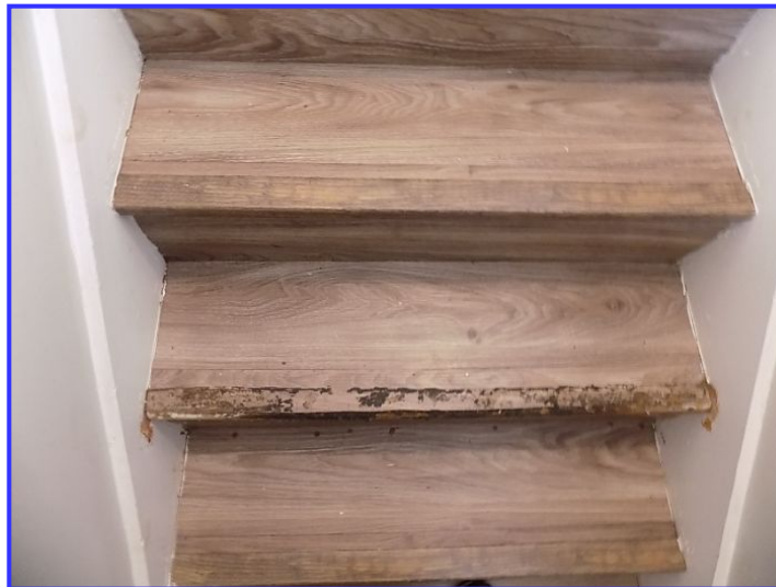
Damage at stars
