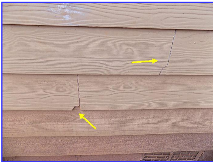
Damaged area of siding at left
