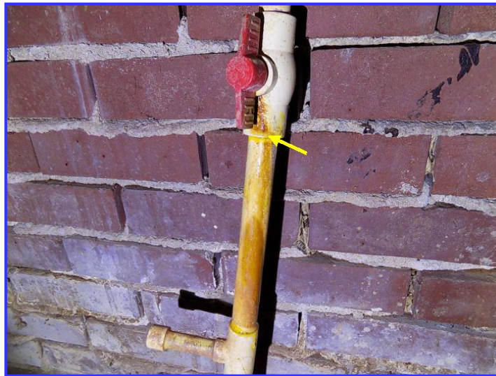
Leak noted at main water shutoff
