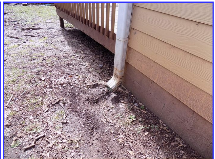
Missing splash block or extension at left side
