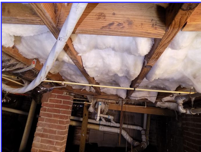
Limited view due to insulation
