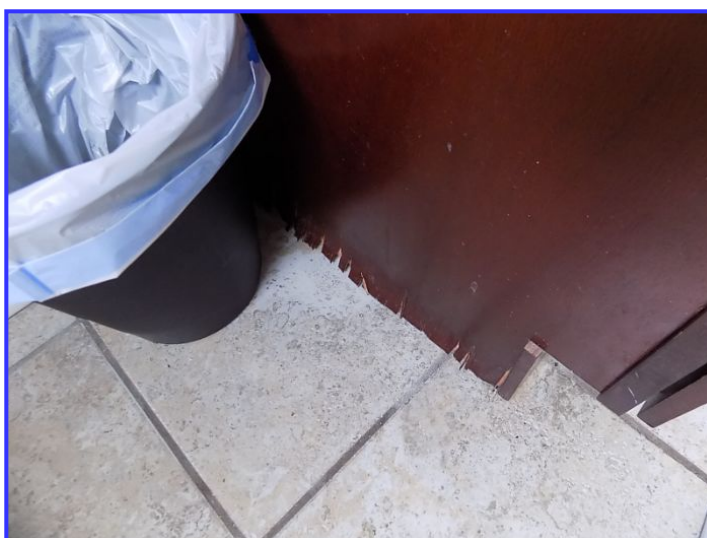
Damaged vanity at upstairs hall bath
