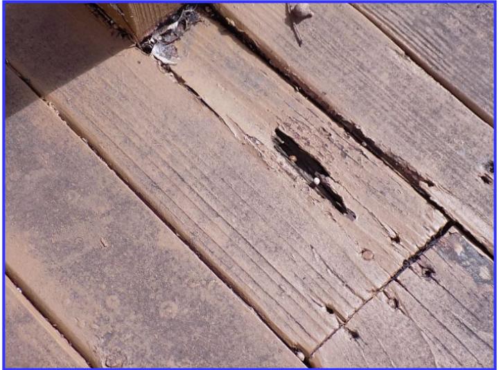
Damaged deck boards noted
