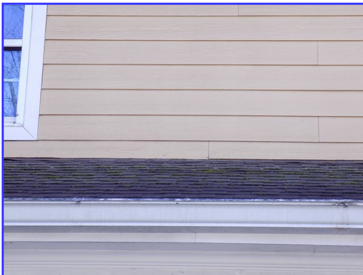
Moss growth at front lower roof
