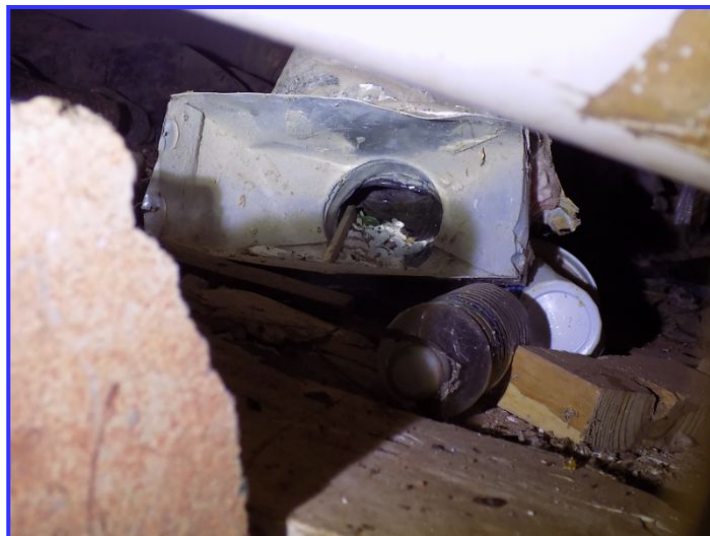
Disconnected duct at left wall
