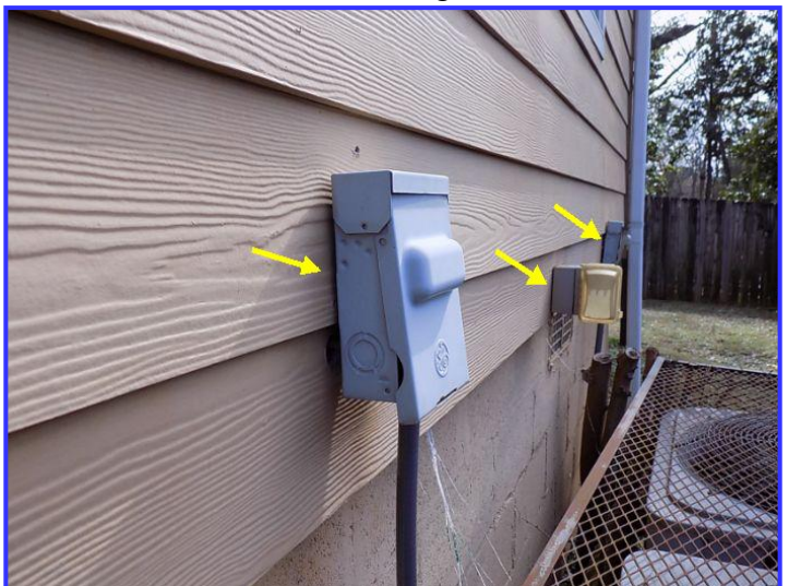
Gap at penetrations at right
