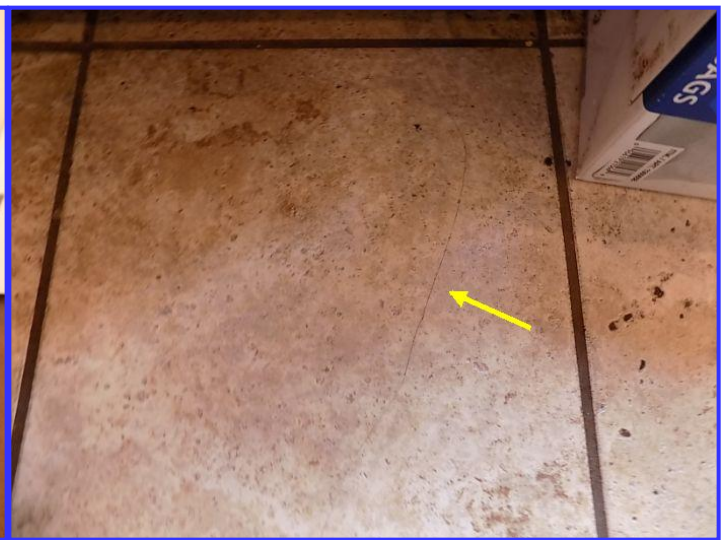
Cracked tiles at kitchen
