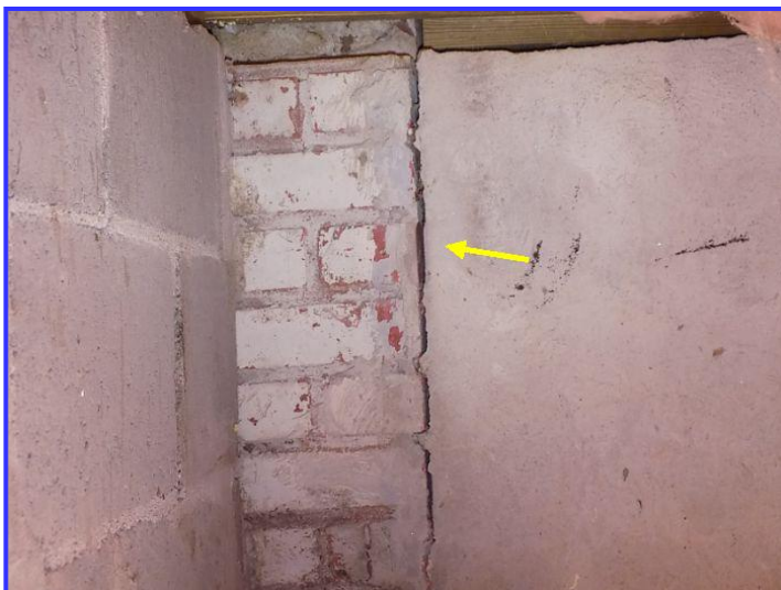
Crack at right wall at brick pier
