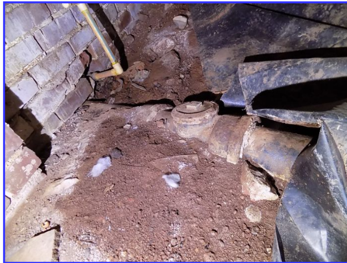
Cast iron/Black steel waste lines noted
