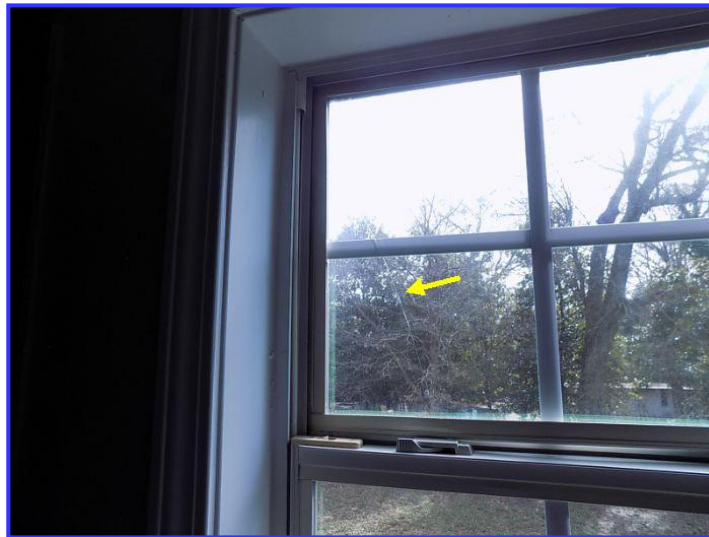
Broken glass at upstairs hall bath
