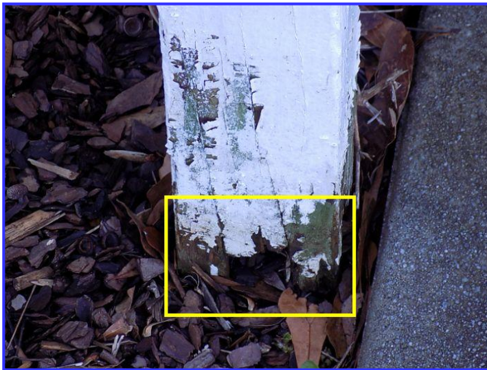
Wood rot at support at front porch
