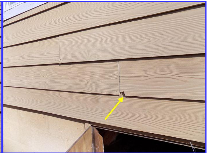
Damaged area of siding at right
