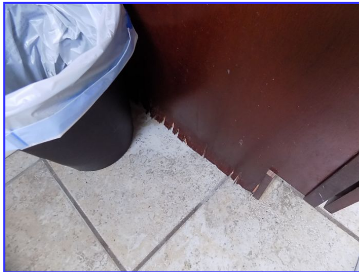
Damaged vanity at upstairs hall bath
