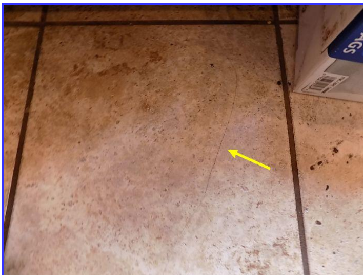
Cracked tiles at kitchen
