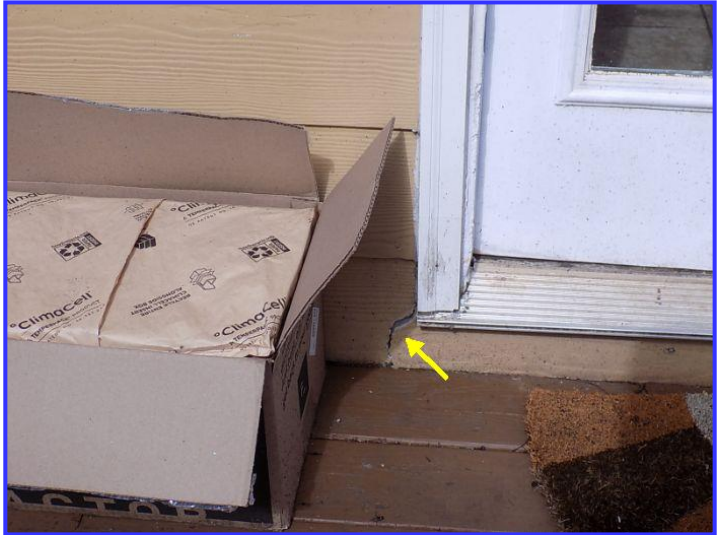
Cracked siding at rear
