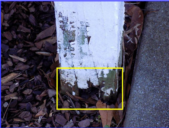
Wood rot at support at front porch
