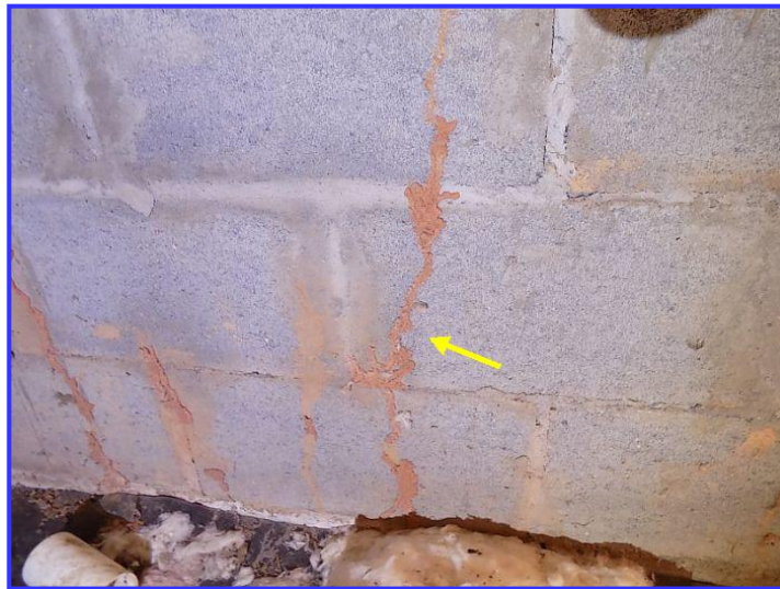
Possible termite activity at right wall
