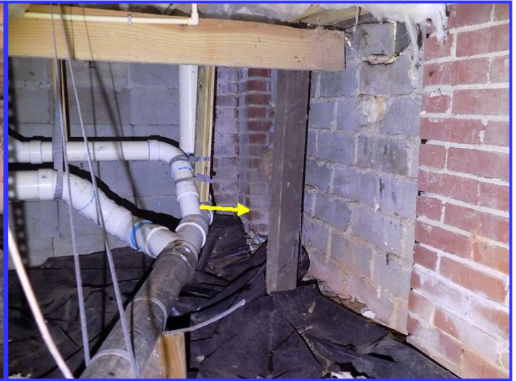
Leaning support at right wall
