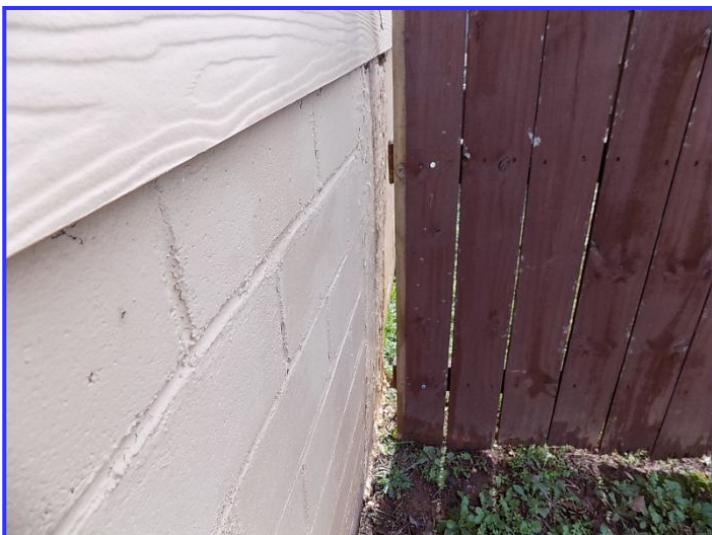
Bulge at foundation section at right side
