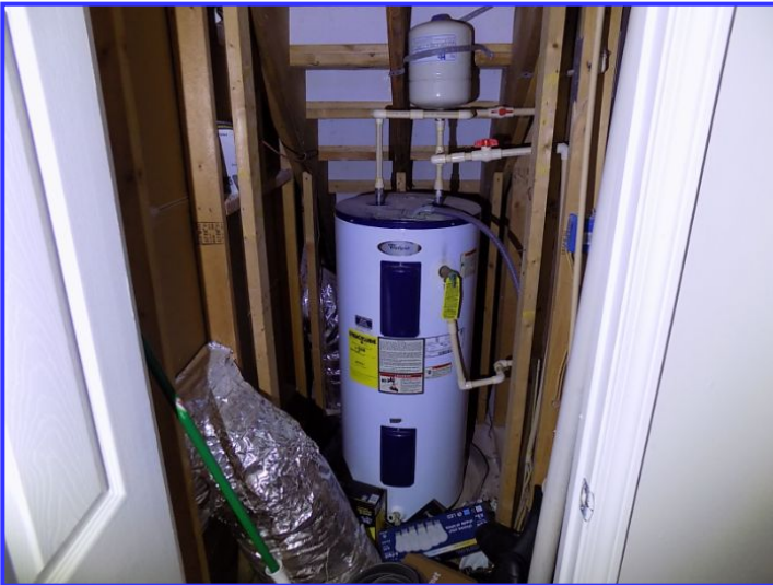
Water heater located in the main level closet
