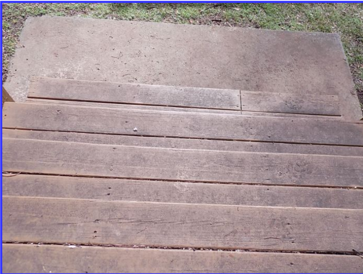
Loose stair treads at rear stairs
