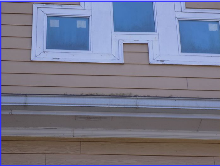
Algae noted at front siding
