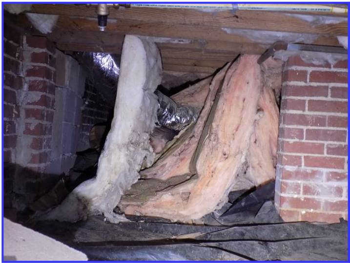
Rodent bored holes in fallen insulation
