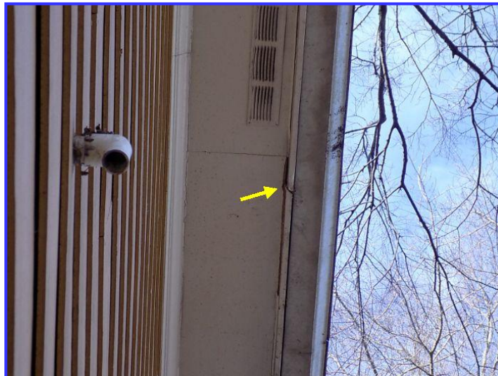
Damaged soffit noted at the left side
