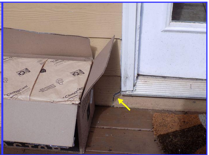
Cracked siding at rear
