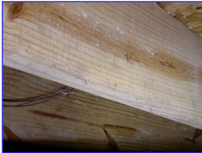
Organic growth on framing
