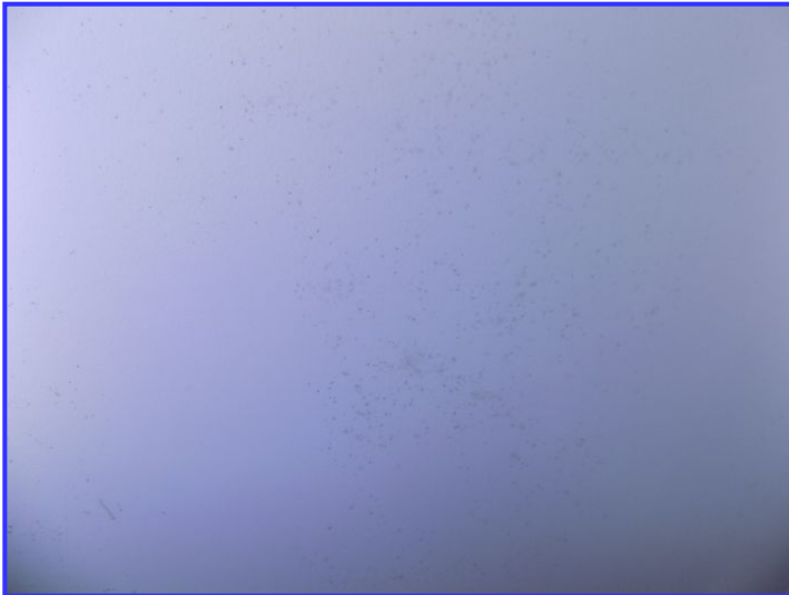
Possible mold/mildew at upstairs hall bath ceiling
