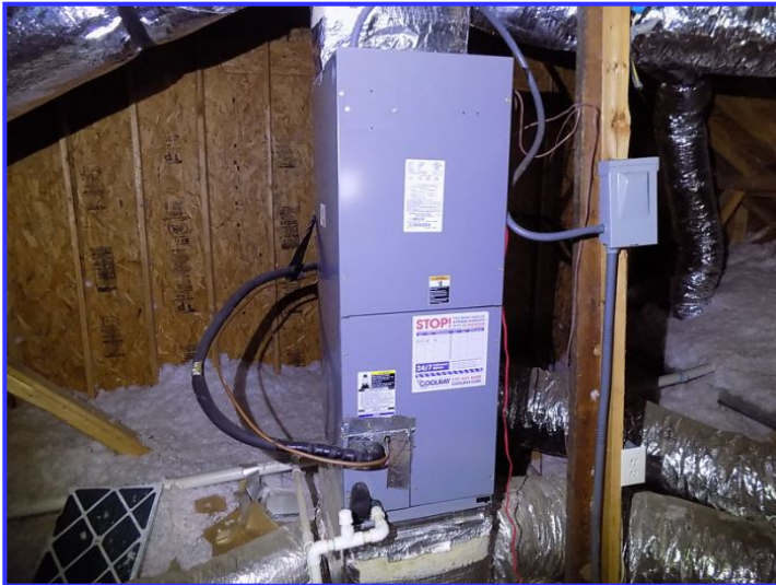
Furnace in Attic
