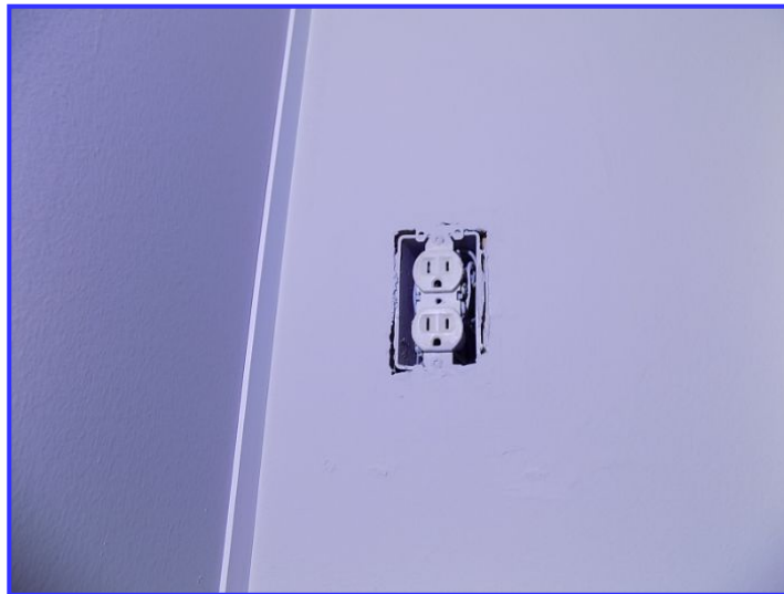
Missing cover plate at unit 3
