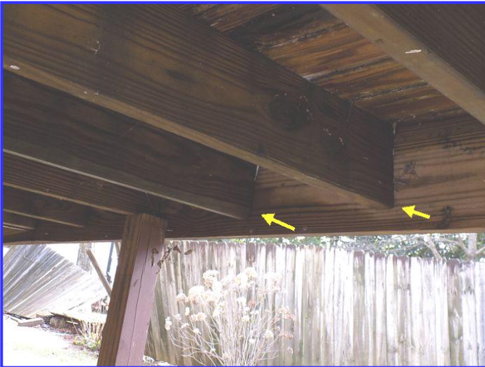
Recommend joist hangers at rear deck
