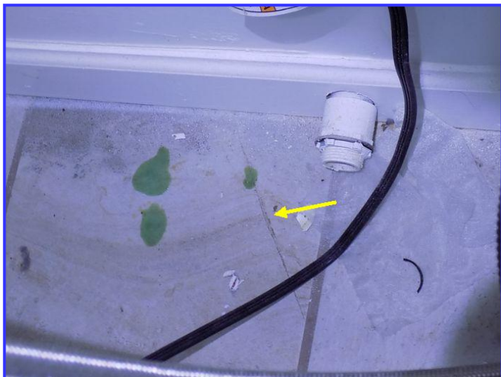
Cracked tiles at laundry room
