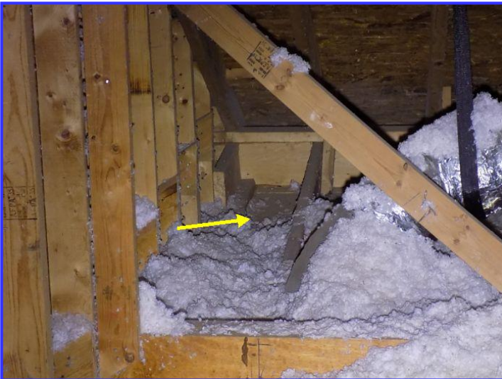
Thin or missing area of insulation in attic
