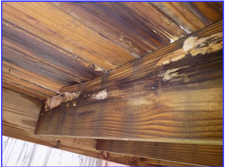
Wood rot at multiple deck joists
