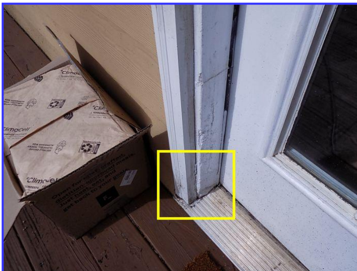
Damaged wood trim at the rear door
