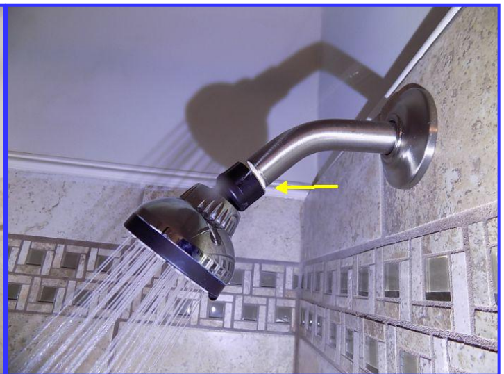
Leak at main level guest bath shower
