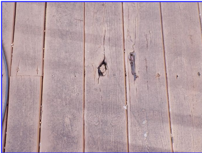
Wood rot at multiple deck boards
