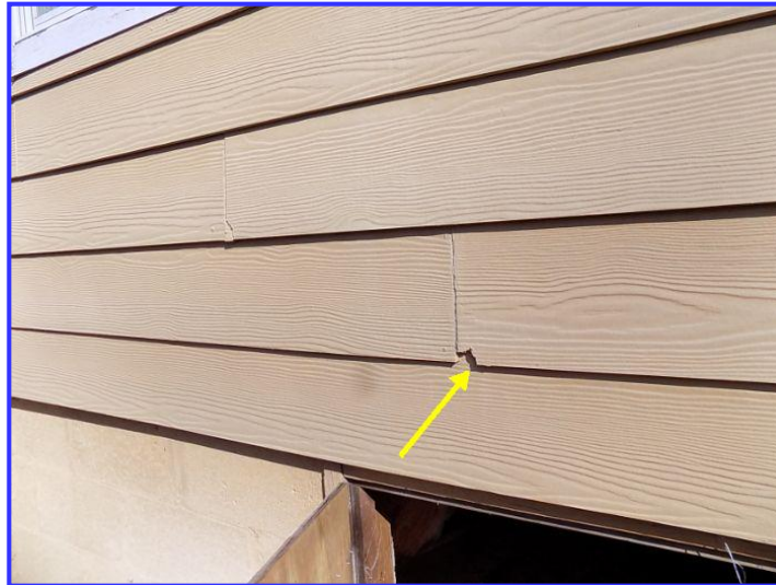
Damaged area of siding at right
