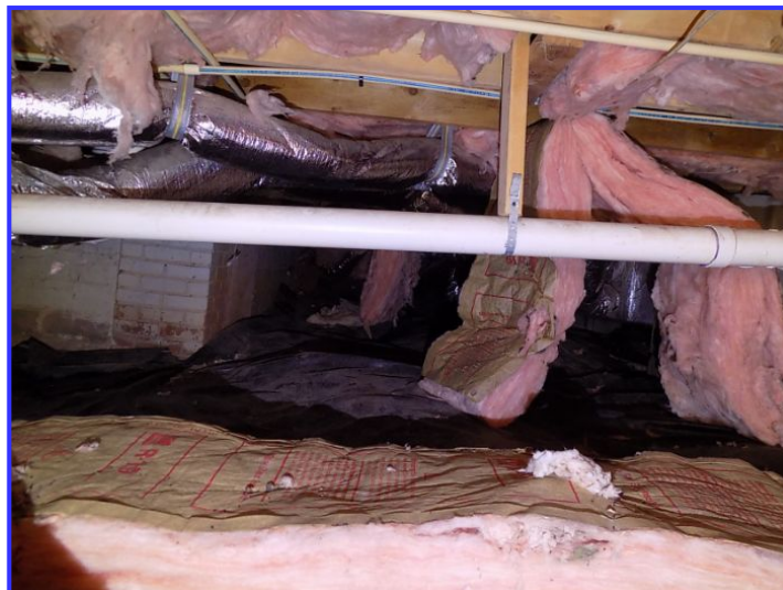
Secure loose insulation at ceiling of crawl space
