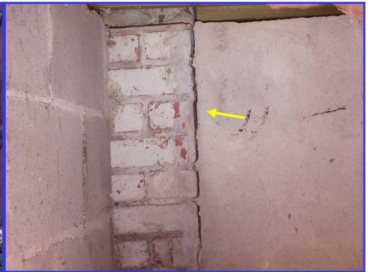
Crack at right wall at brick pier
