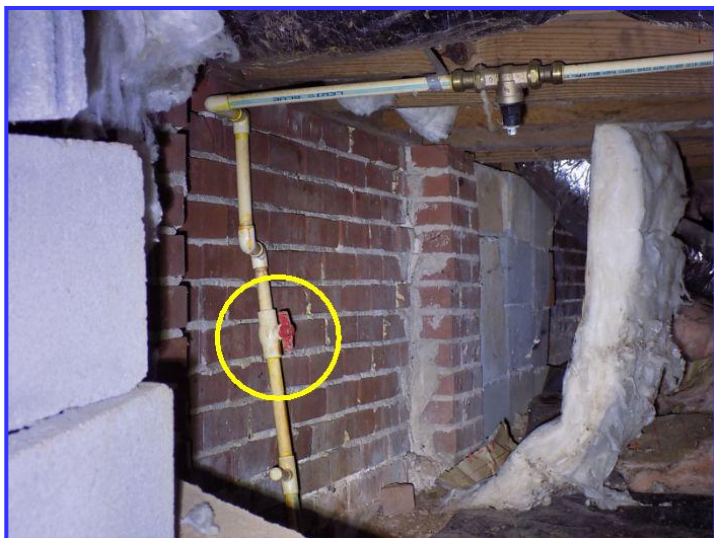
Main water shut off noted at the front crawl space wall
