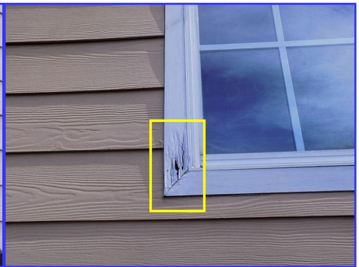
Damaged window framing at right side
