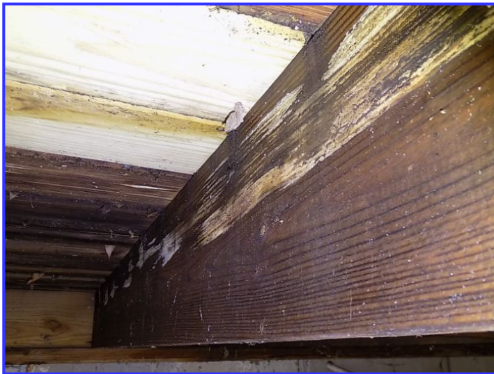
Wood rot at multiple deck joists
