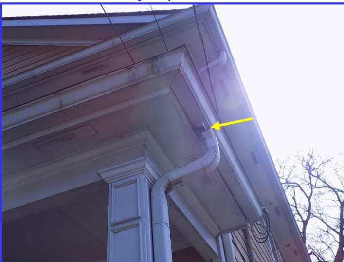
Disconnected gutter at front right
