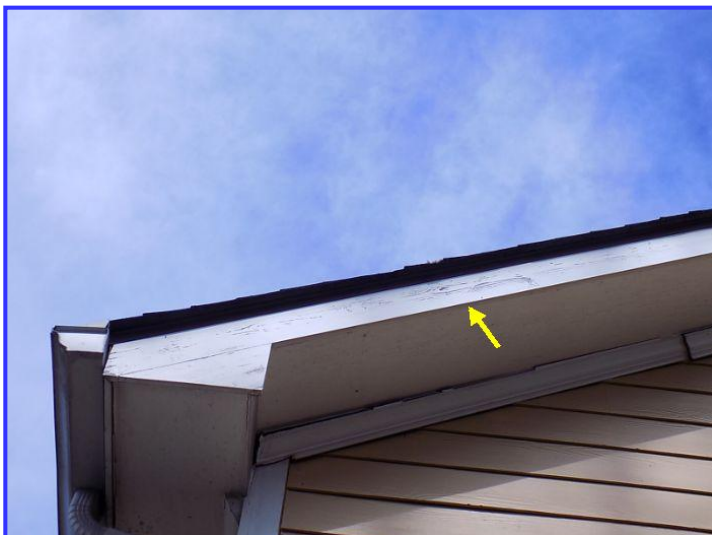
Weathered fascia at rear
