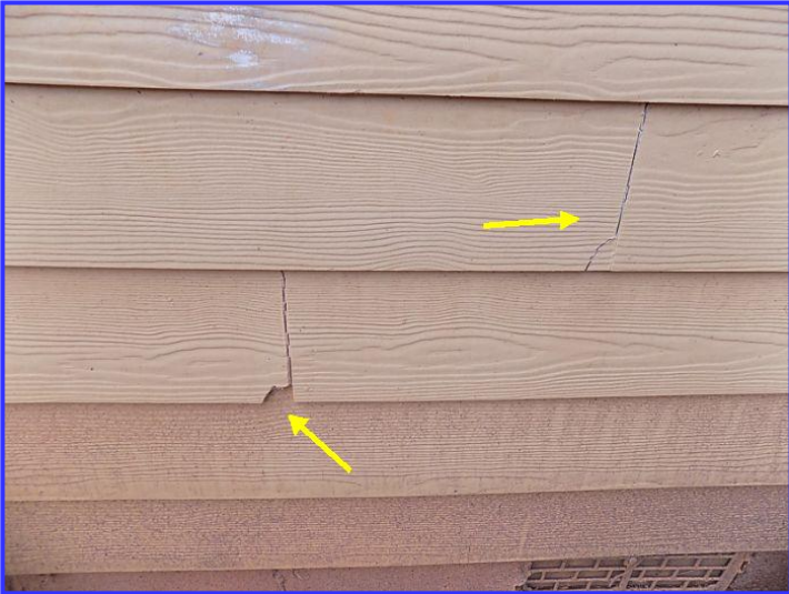
Damaged area of siding at left
