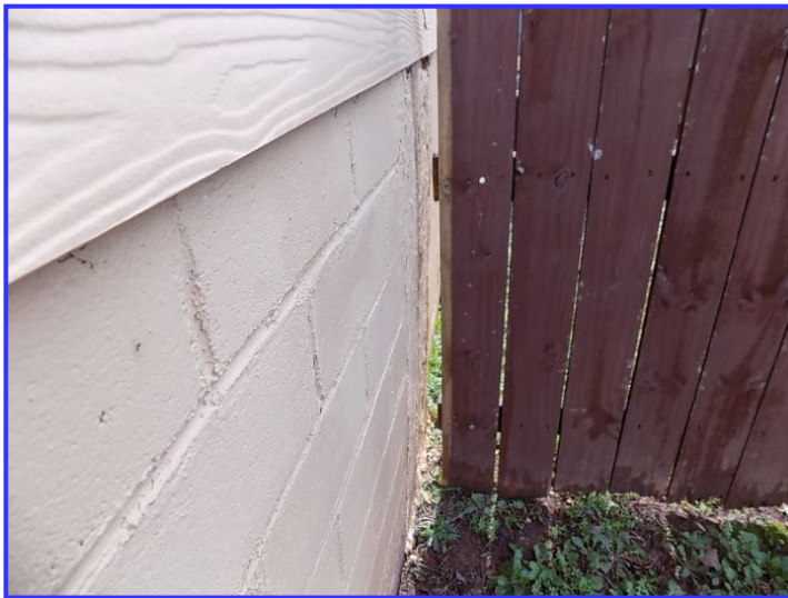
Bulge at foundation section at right side
