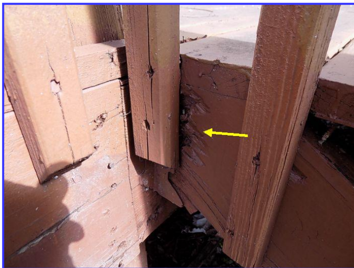
Stringer rot at rear deck
