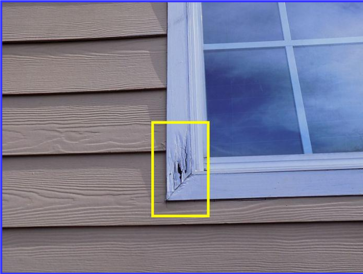
Damaged window framing at right side
