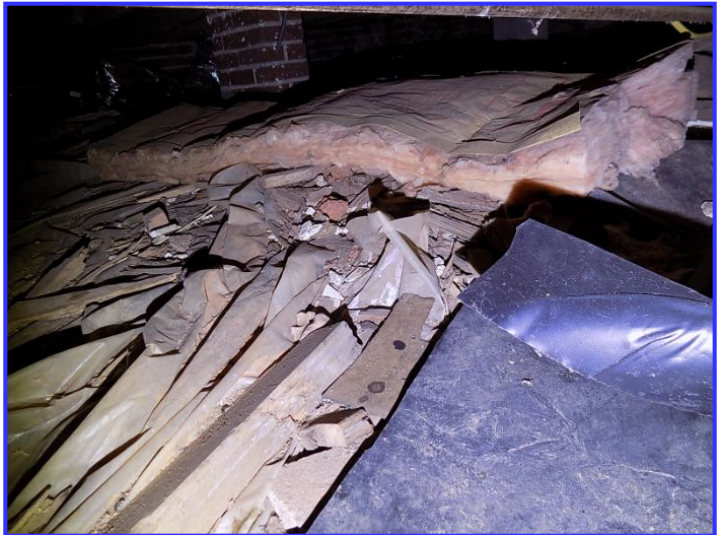
Wood debris noted
