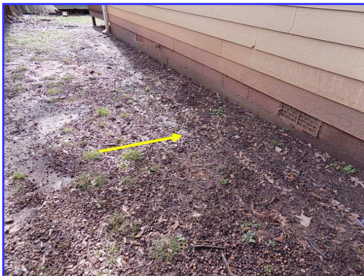
Poor slope at the left side
