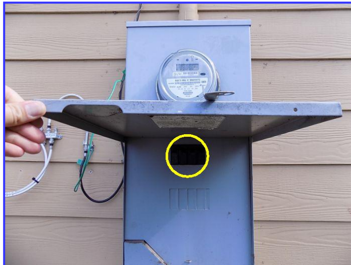
Electric meter and 200 amp shut off at the right side
