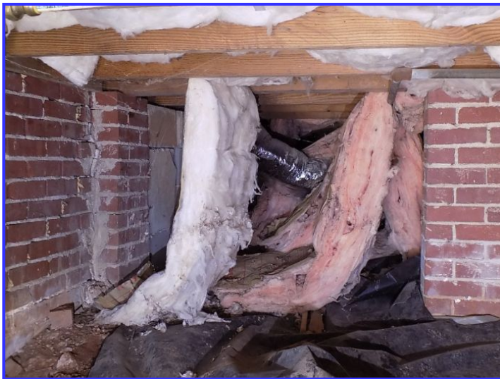
Limited view at front wall due to fallen insulation
