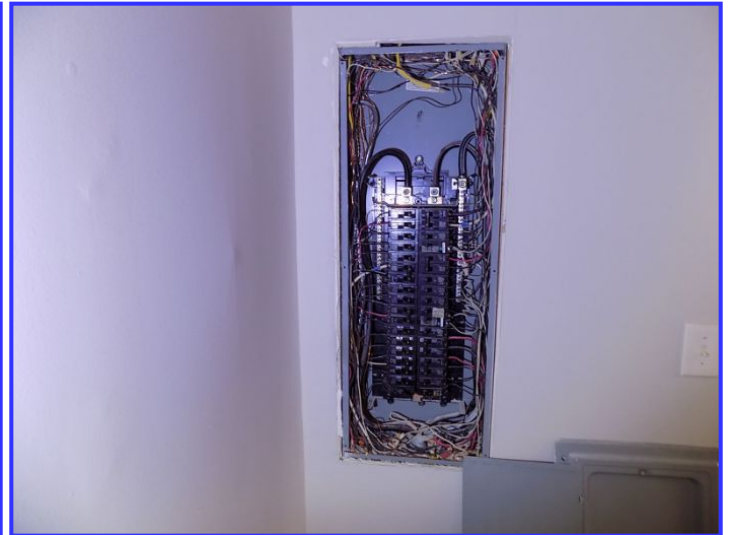
Interior wiring at main panel
