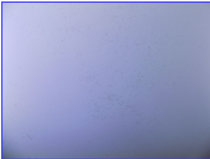
Possible mold/mildew at upstairs hall bath ceiling
