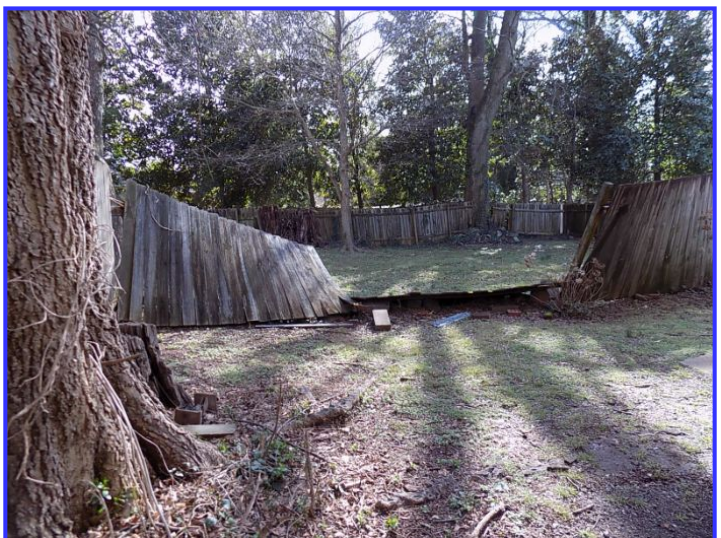
Damaged fence noted
