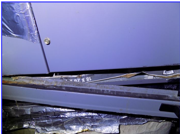
Filter located in the lower portion/side of the furnace(s)
