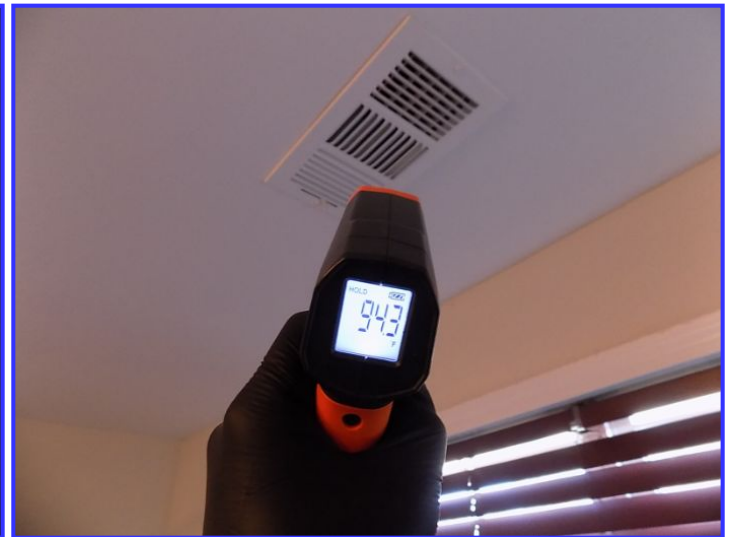
Heat Temperature (Second Floor)
