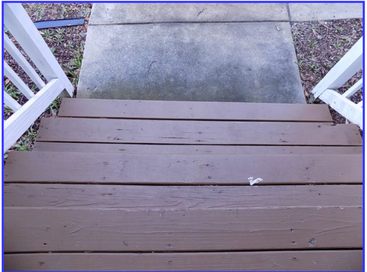
Loose stair treads at front
