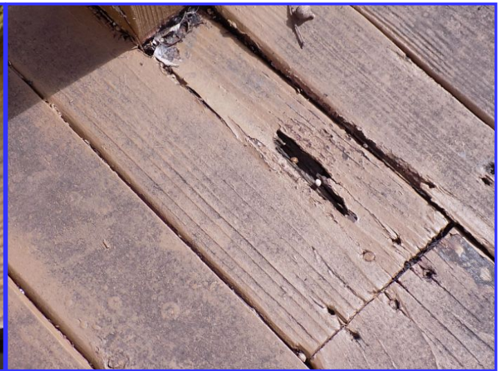
Damaged deck boards noted
