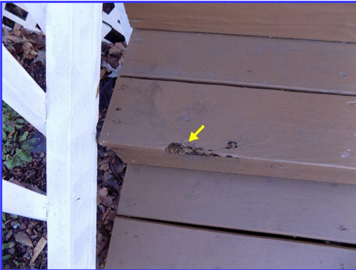
Damaged tread at front porch stairs
