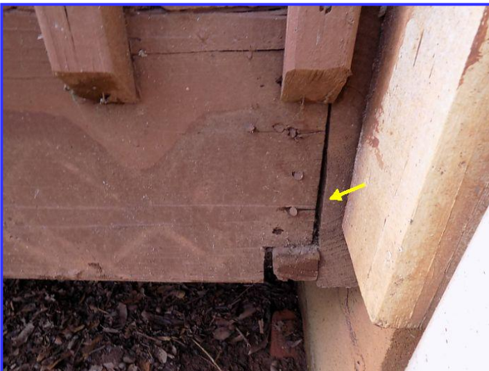
Separation at band at rear deck
