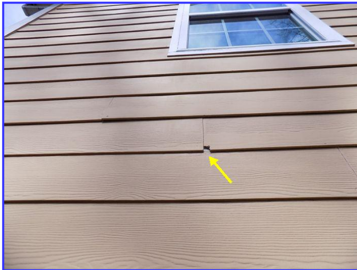
Damaged area of siding at rear
