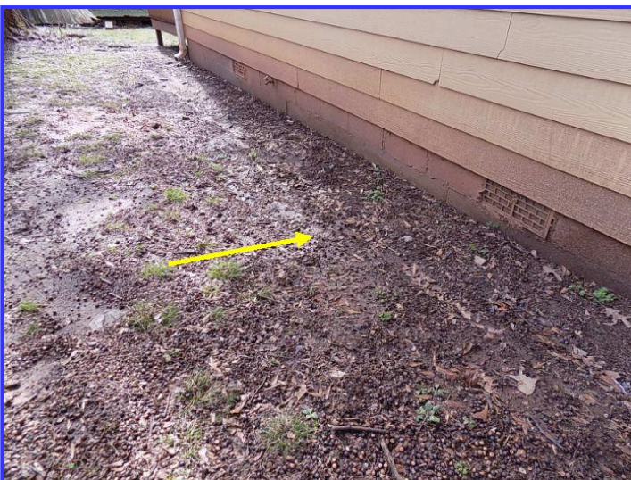
Poor slope at the left side
