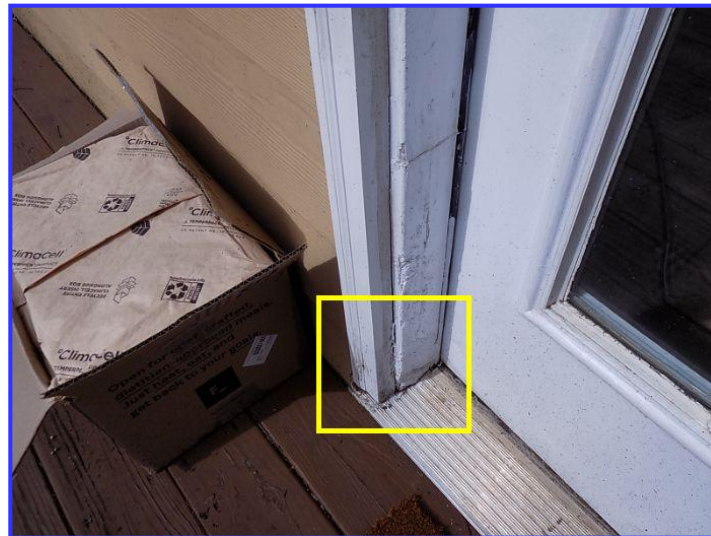
Damaged wood trim at the rear door
