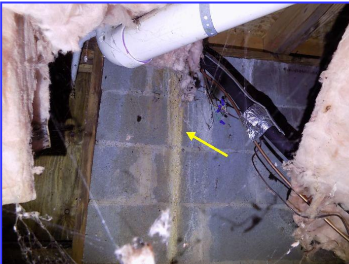
Efflorescence noted at rear wall
