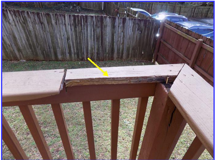
Damaged handrail at rear deck
