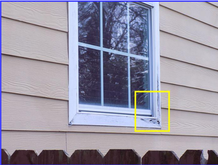
Damaged window framing at right
