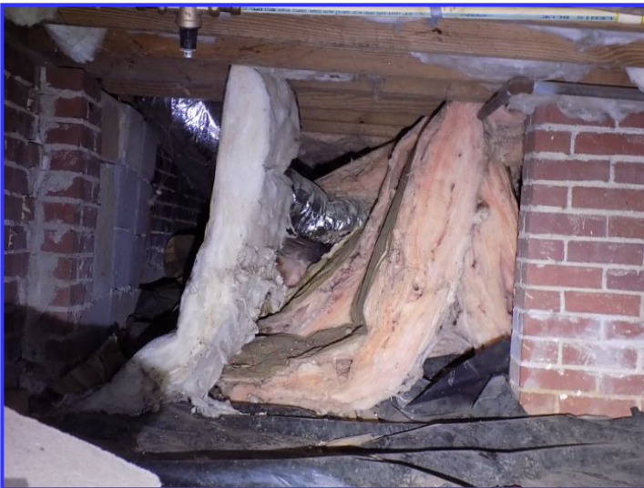
Rodent bored holes in fallen insulation
