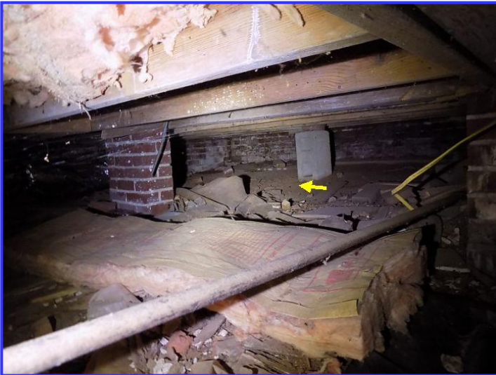
Gap at vapor barrier at front left wall
