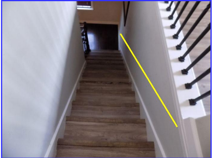
Recommend handrail at stairs
