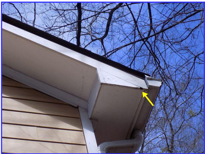
Damaged fascia at the rear left corner
