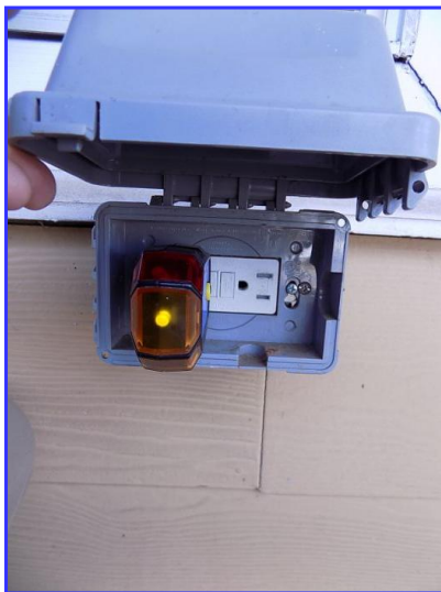
GFCI will not trip when tested at front
