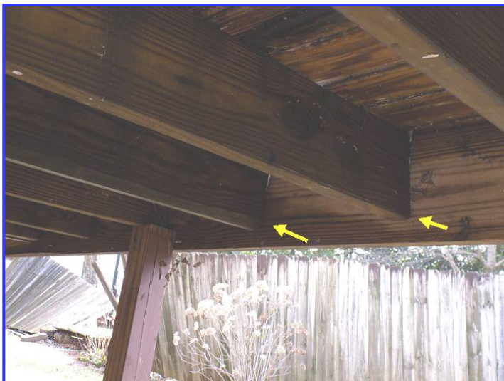
Recommend joist hangers at rear deck
