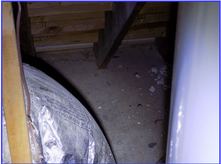
Rodent droppings under stairs at main level
