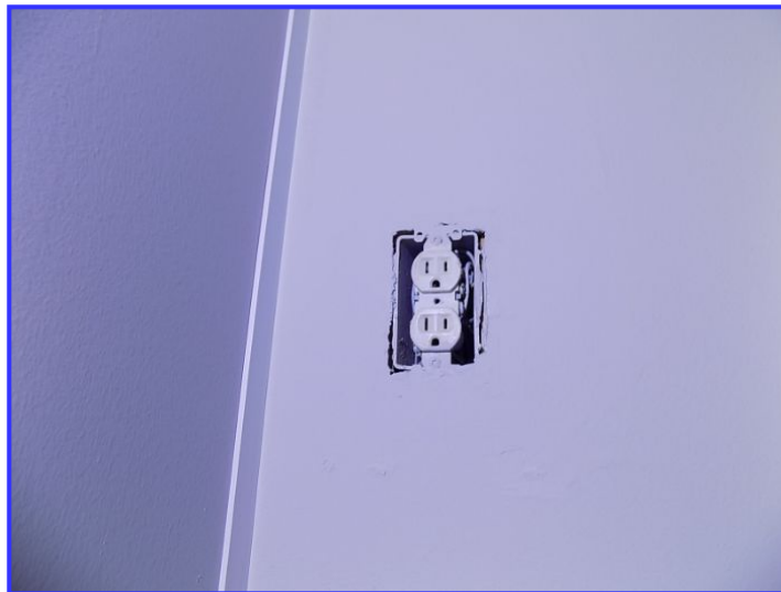
Missing cover plate at unit 3
