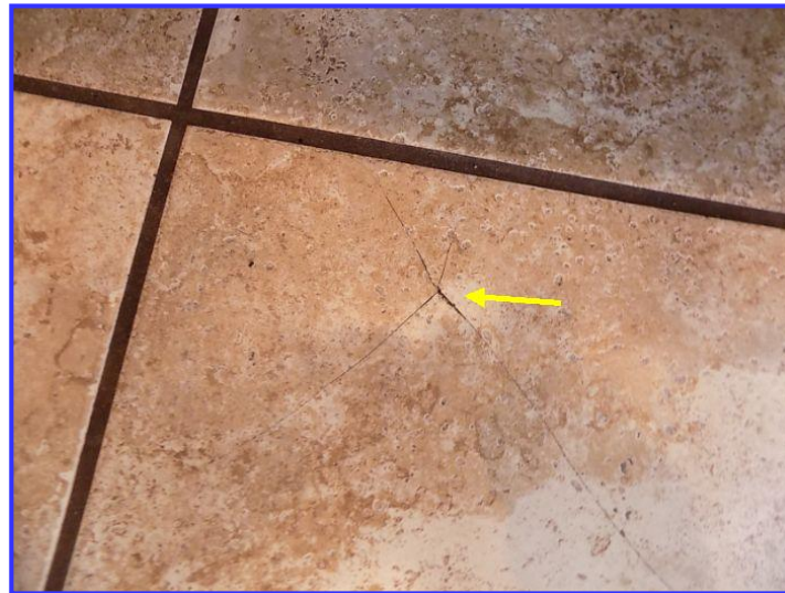
Cracked tiles at kitchen
