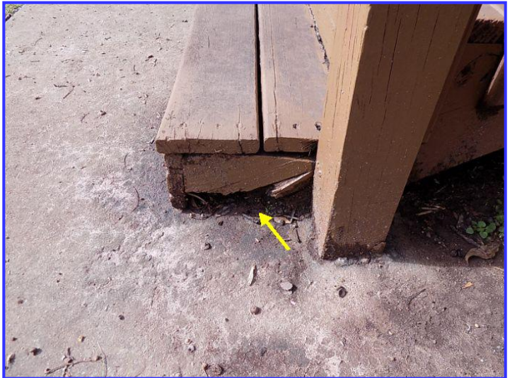
Water damaged stringer at rear deck stairs
