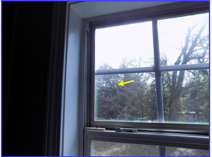
Broken glass at upstairs hall bath
