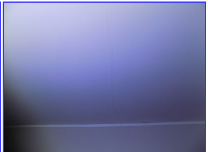
Crack at ceiling at unit 4
