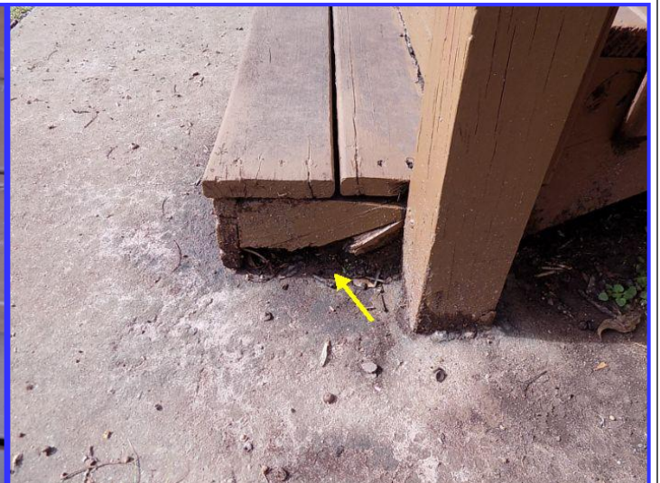
Water damaged stringer at rear deck stairs
