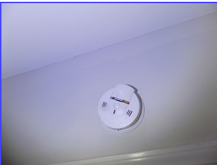
Missing battery at smoke detector in kitchen
