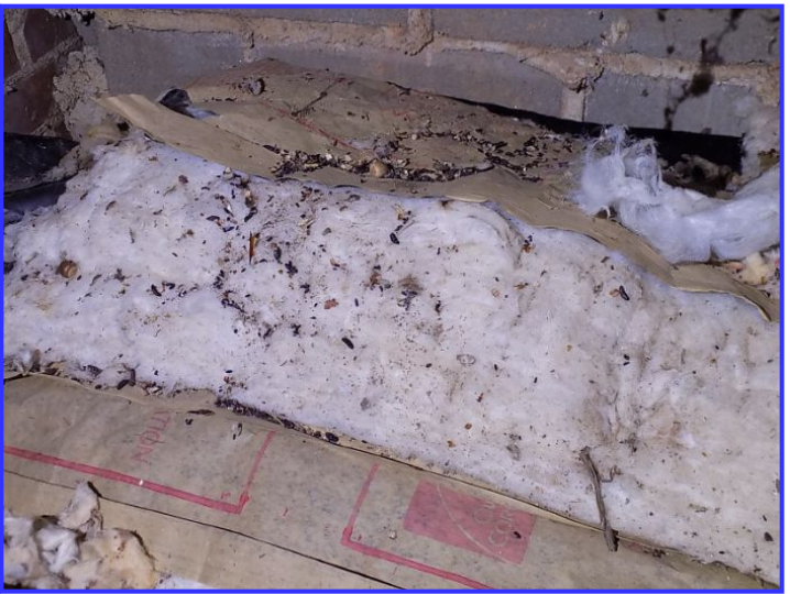
Rodent contaminated insulation in crawlspace
