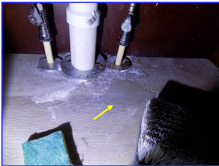
Leak at drain under sink in the upstairs hall bath
