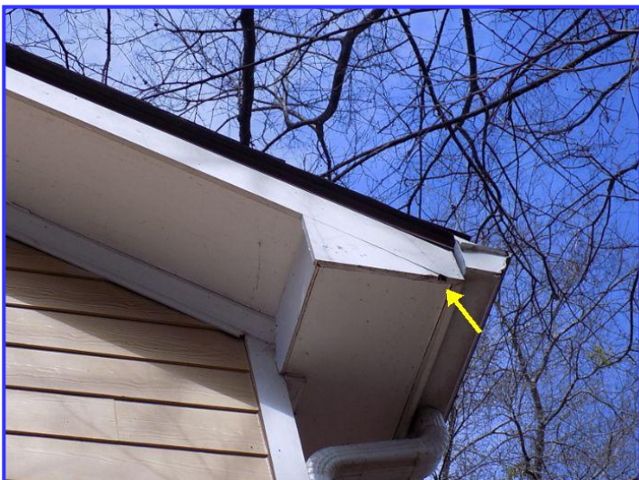
Damaged fascia at the rear left corner
