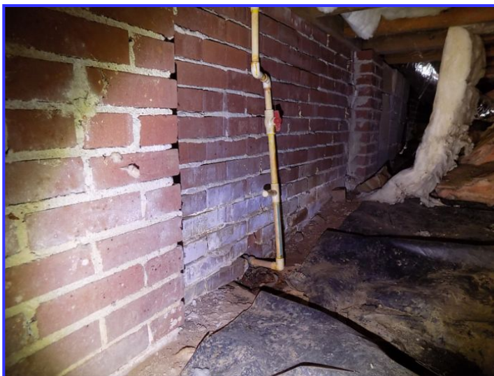
Main water line
