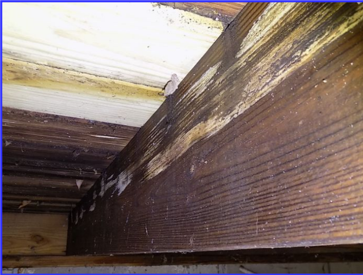
Wood rot at multiple deck joists
